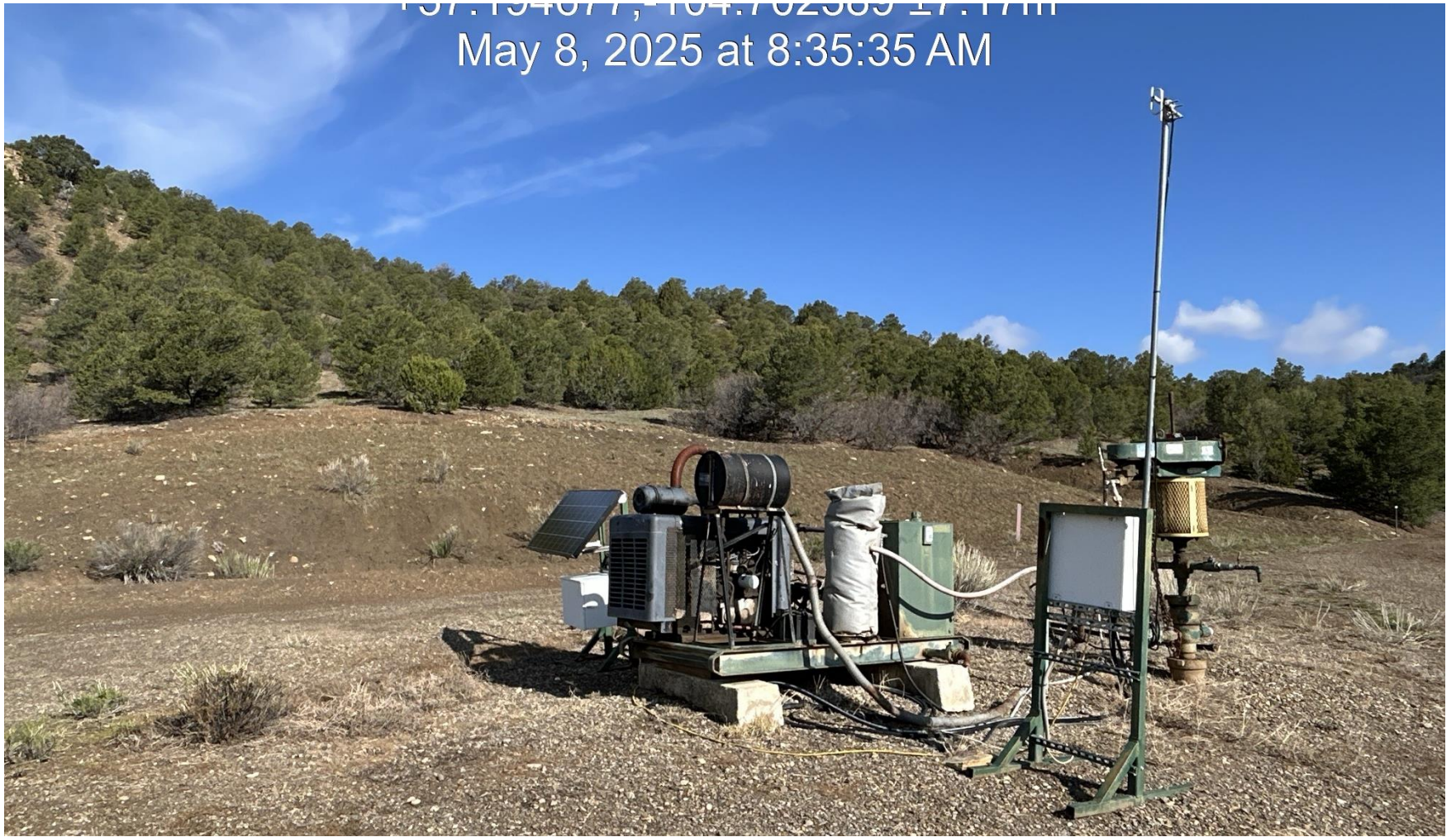
PHOTO 3: WELLHEAD AND EQUIPMENT
