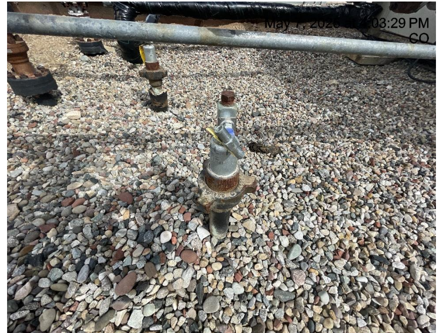
Photo # 9645 Unused flowline lacks lockout tagout (OOSLAT)
