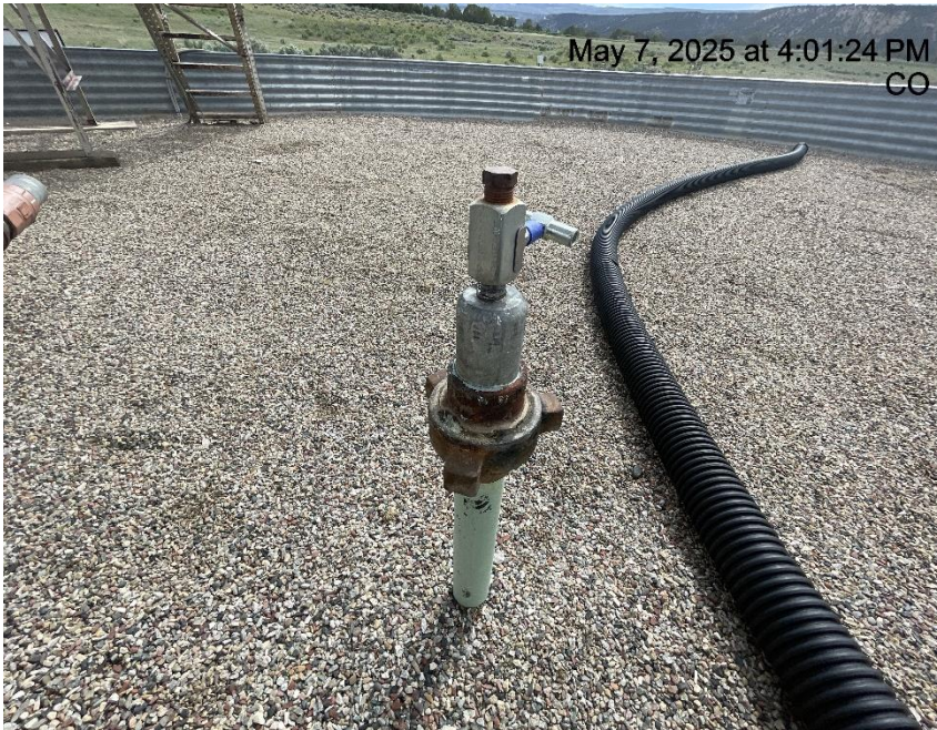
Photo # 9644 Unused flowline lacks lockout tagout (OOSLAT)
