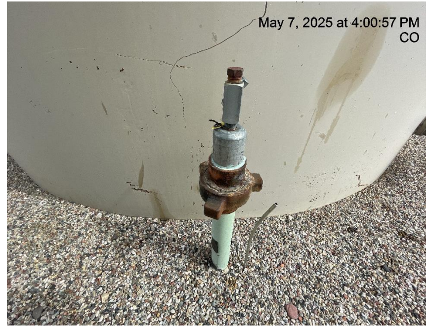
Photo # 9643 Unused flowline lacks lockout tagout (OOSLAT)
