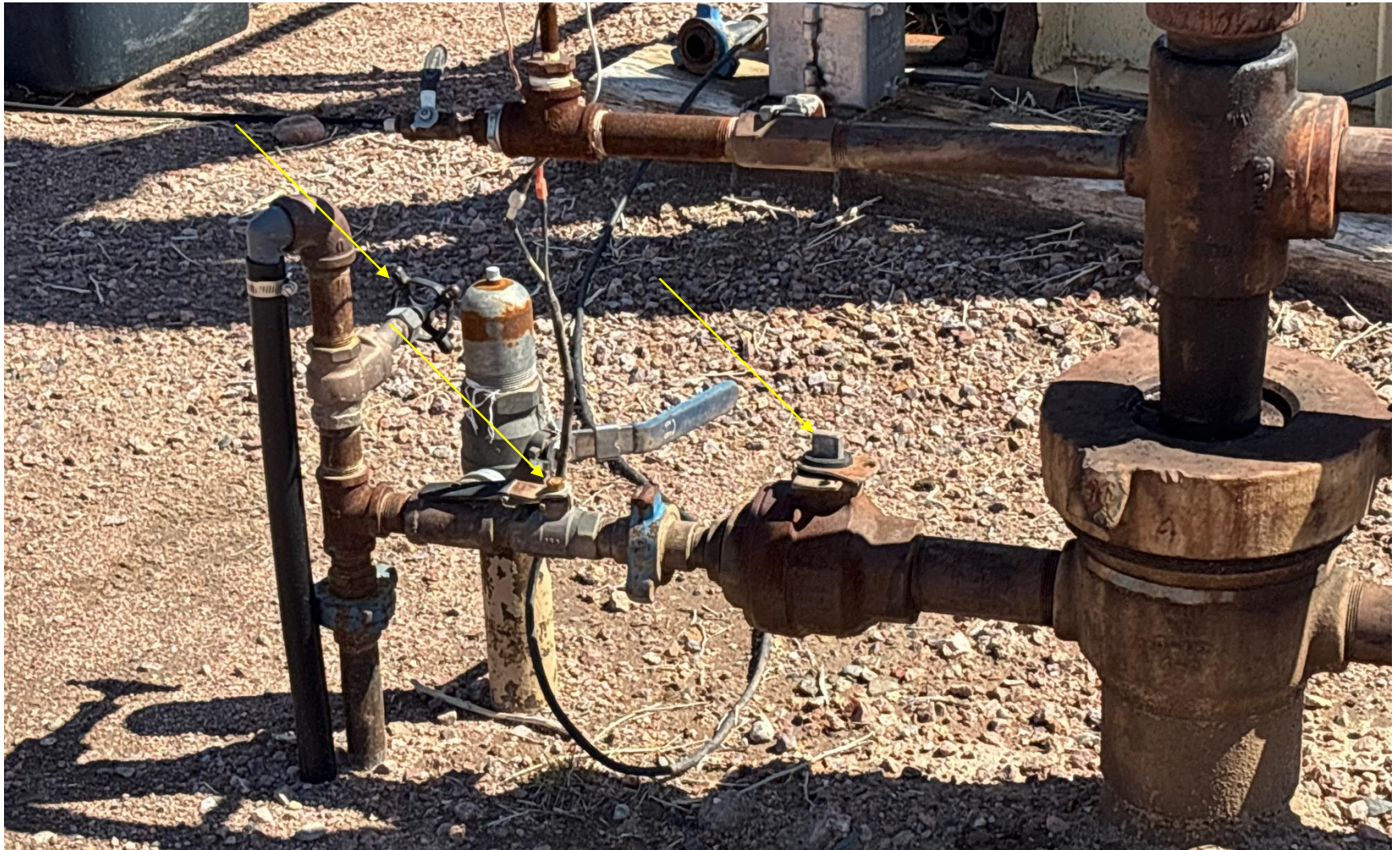
PHOTO 5: TBG/CSG ANNULUS IS PLUMBED TO CRUDE OIL TANK BATTERY AND VALVES APPEAR TO BE OPEN.
