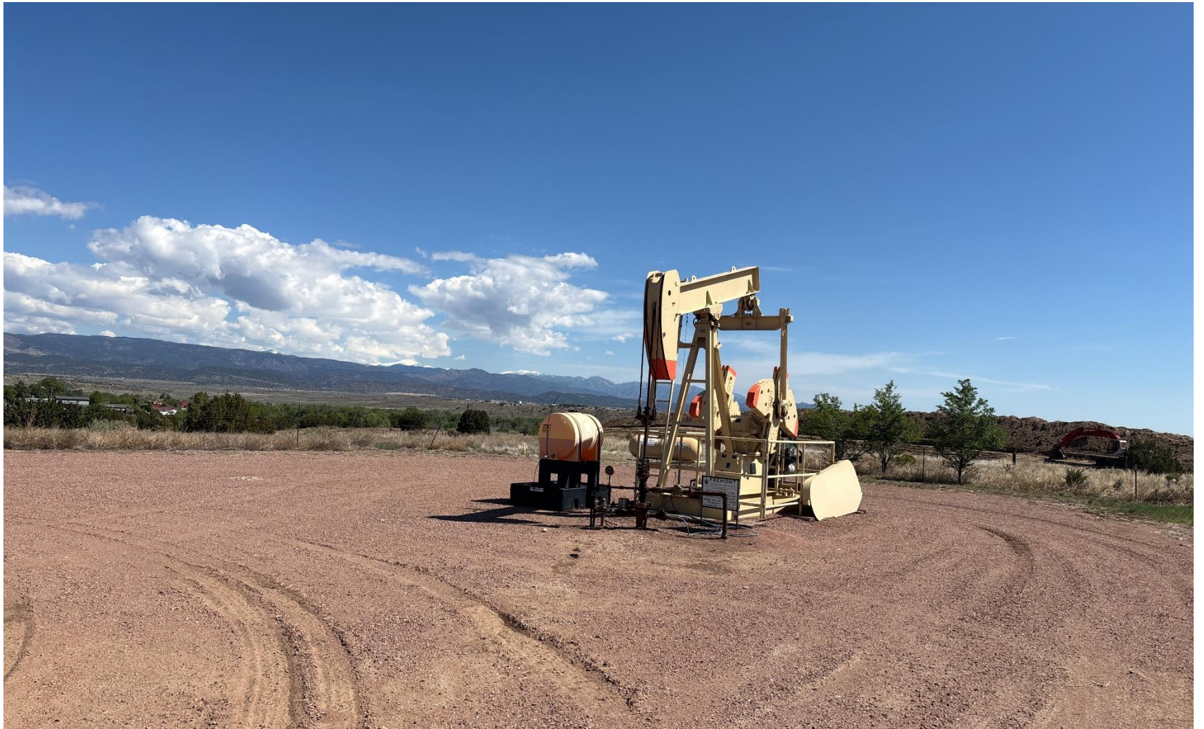
PHOTO 3: WELLHEAD AND EQUIPMENT.
