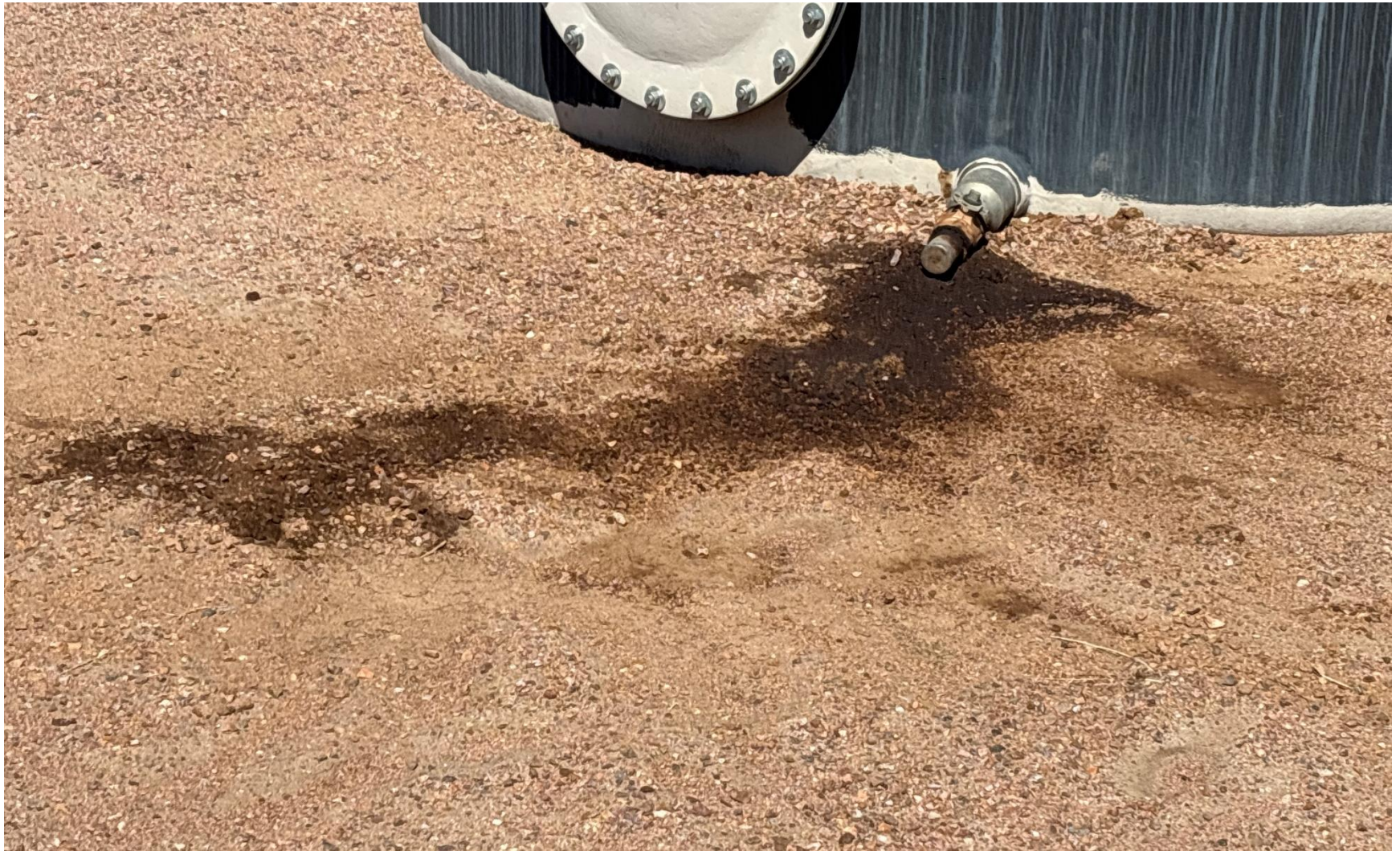
PHOTO 7: THERE IS AN AREA OF IMPACTED SOIL ON BACKSIDE OF TANK BATTERY NEAR 2" VALVE. Conduct maintenance on equipment, cleanup stained material and review self inspection processes. COMPLY WITH RULE 1002,(2).D CA DATE 5/21/2025.
