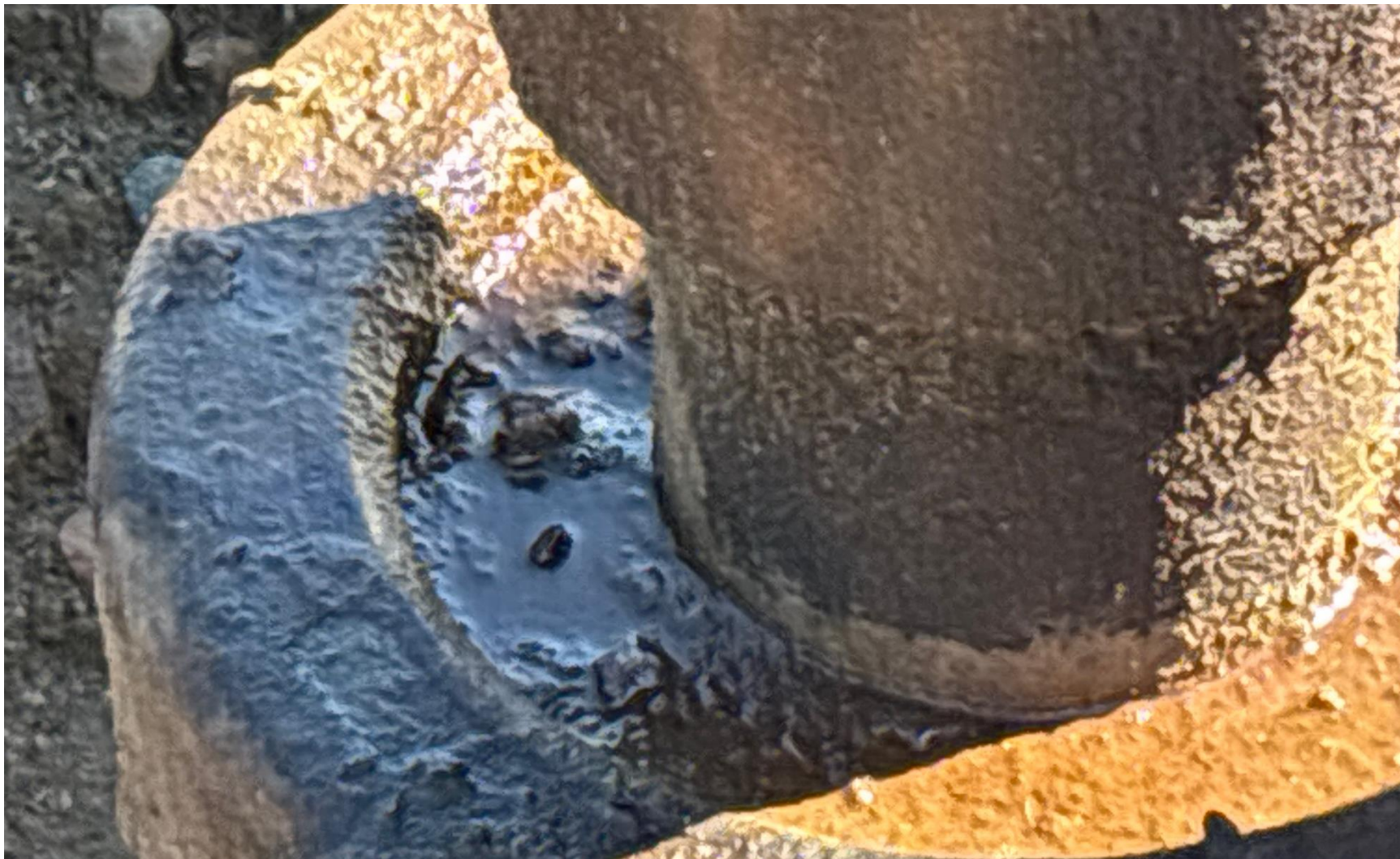
PHOTO 6: Mechanical issue well head leaking around tubing nut see video. Securely fasten all valves, pipes, fittings, and Production Facilities to ensure good mechanical condition, inspect at regular intervals and maintain in good mechanical condition per Rule 608.e.. THIS IS THE SECOND NOTICE, IMMEDIATE ACTION IS REQUIRED.
