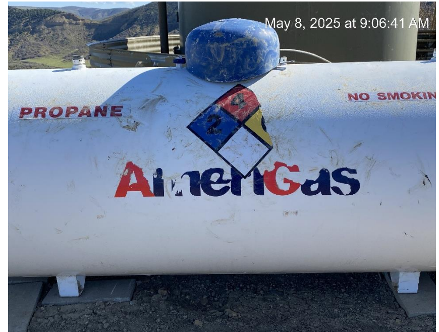
Replace damaged or illegible labels
