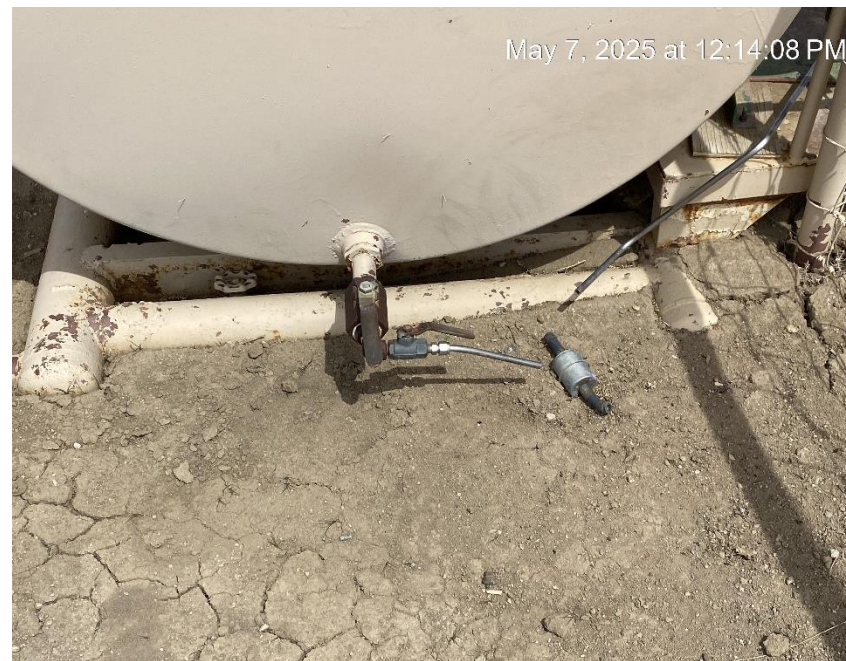
Empty. Disconnected. Unused equipment.
