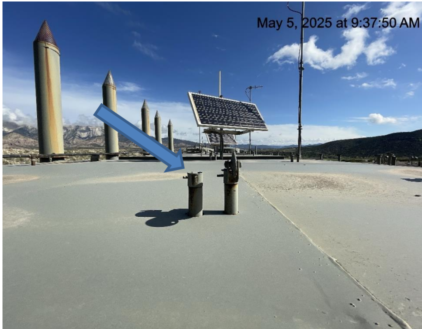
Photo # 8653 PRV vent line does not comply with CECMC pressure safety device rules
