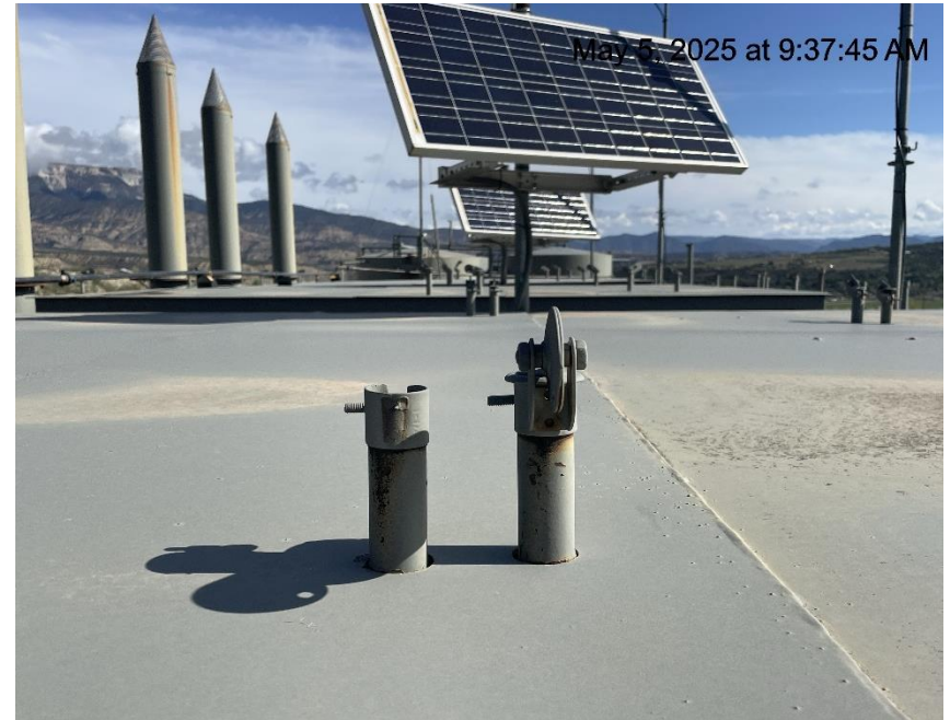
Photo # 8654 PRV vent line does not comply with CECMC pressure safety device rules
