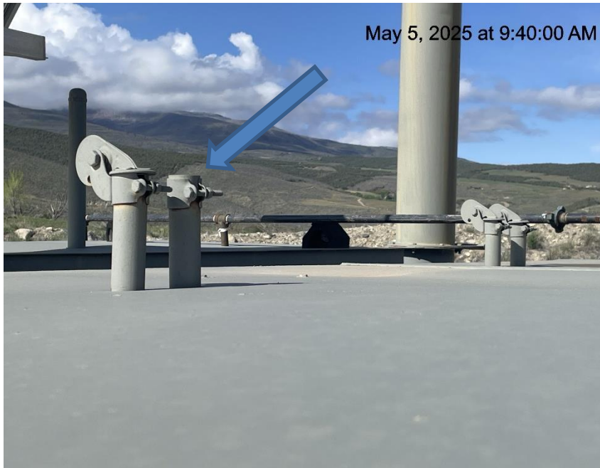
Photo # 8655 PRV vent line does not comply with CECMC pressure safety device rules
