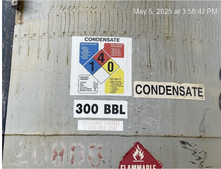
Incomplete tank label
