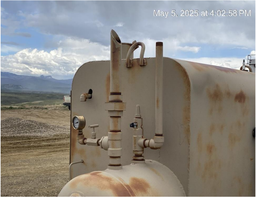
Unprotected relief vents
