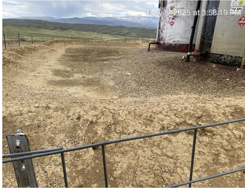
Tank berm insufficient
