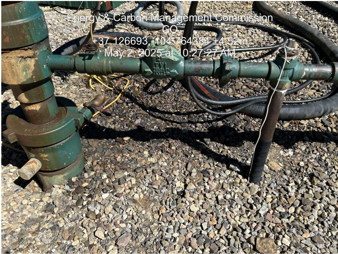
PHOTO 4: Impacted soil from voac leak
