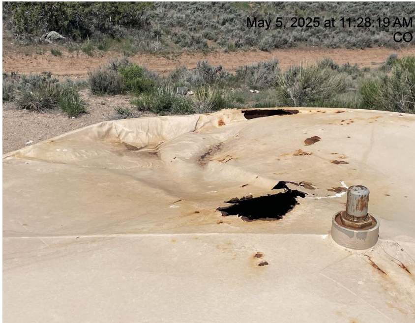
Photo # 8903 Tank failure – Multiple holes in 210 bbl production tank/tank lacks integrity (Additionally the holes also constitute a wildlife hazard)
