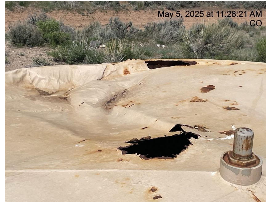
Photo # 8904 Tank failure – Multiple holes in 210 bbl production tank/tank lacks integrity (Additionally the holes also constitute a wildlife hazard)
