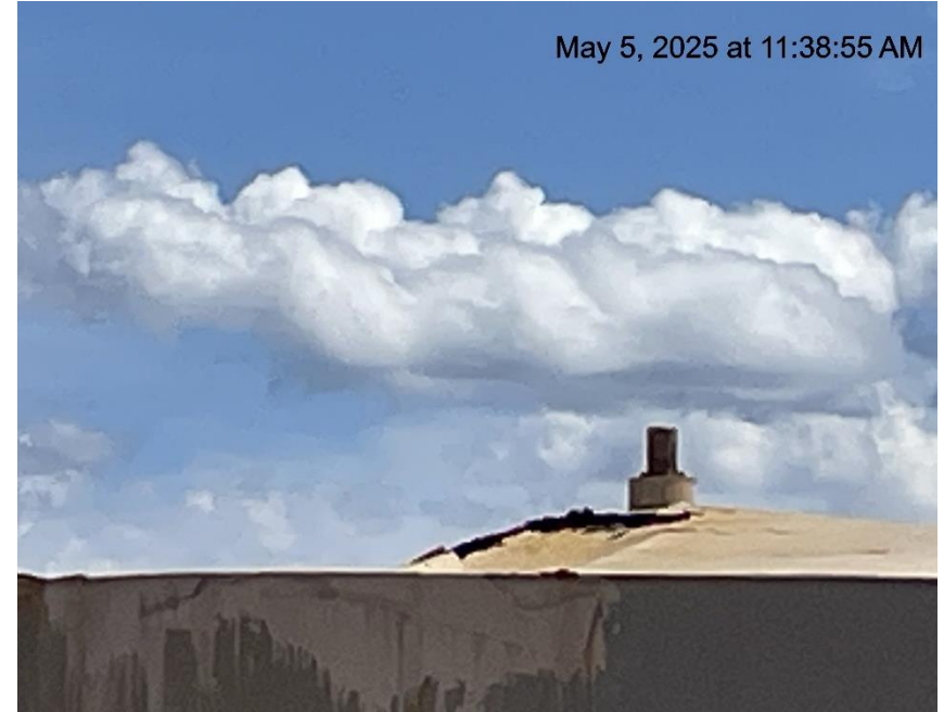
Photo # 8908 Tank failure – Multiple holes in 210 bbl production tank/tank lacks integrity (Additionally the holes also constitute a wildlife hazard)
