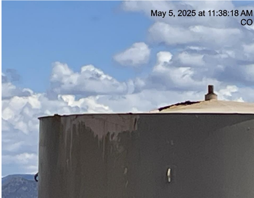
Photo # 8907 Tank failure – Multiple holes in 210 bbl production tank/tank lacks integrity (Additionally the holes also constitute a wildlife hazard)
