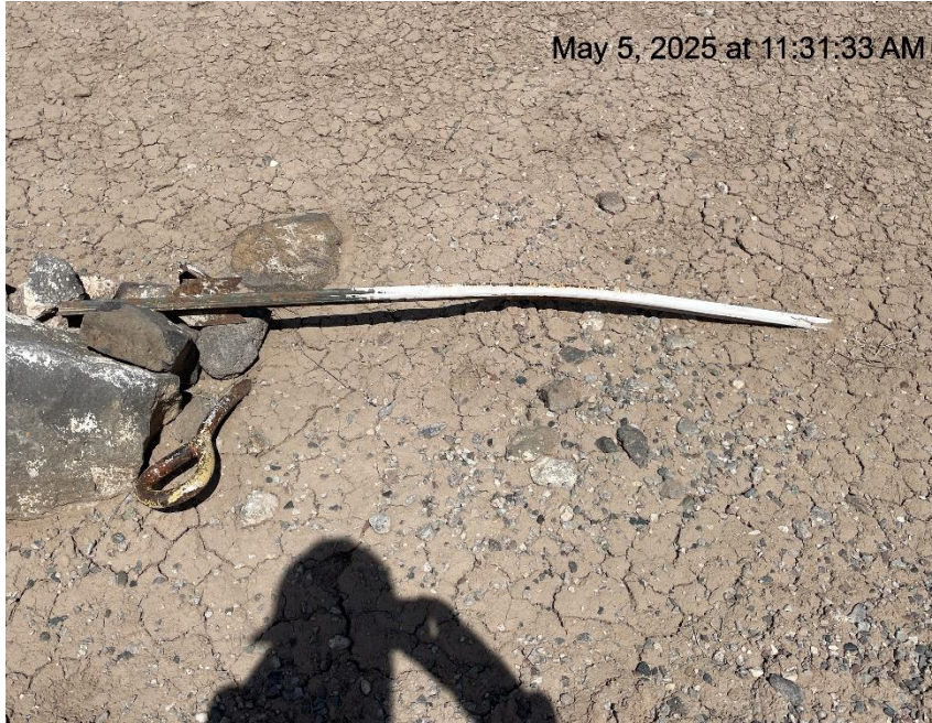
Photo # 8911 Improperly marked deadman
