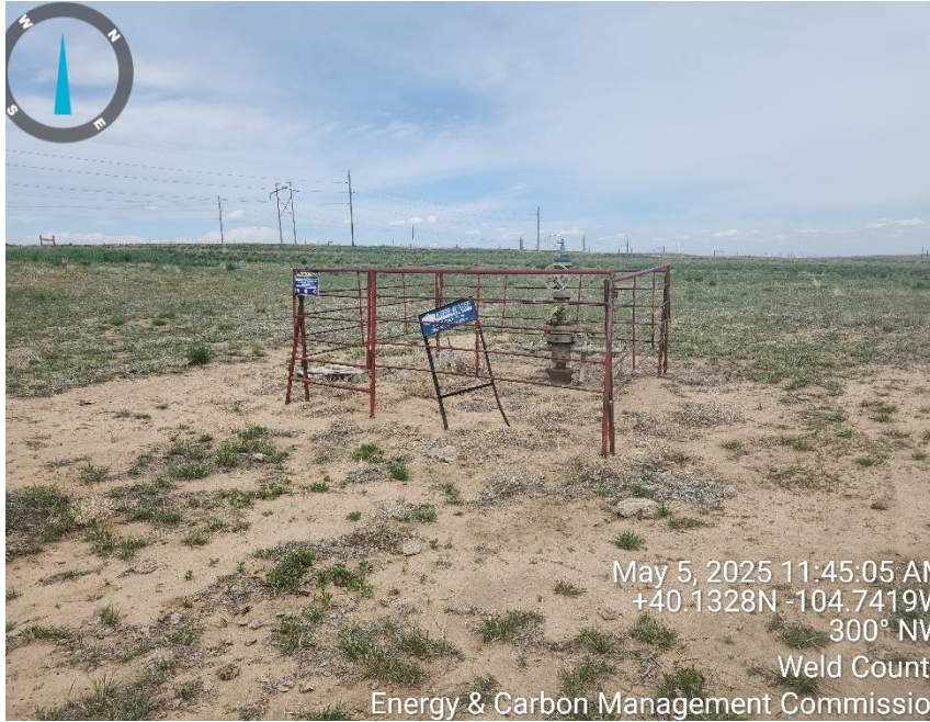
Photo 1 well head and equipment
