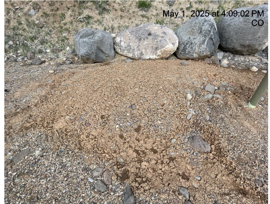
Photo # 8383 Stockpiled soils with no BMP's
