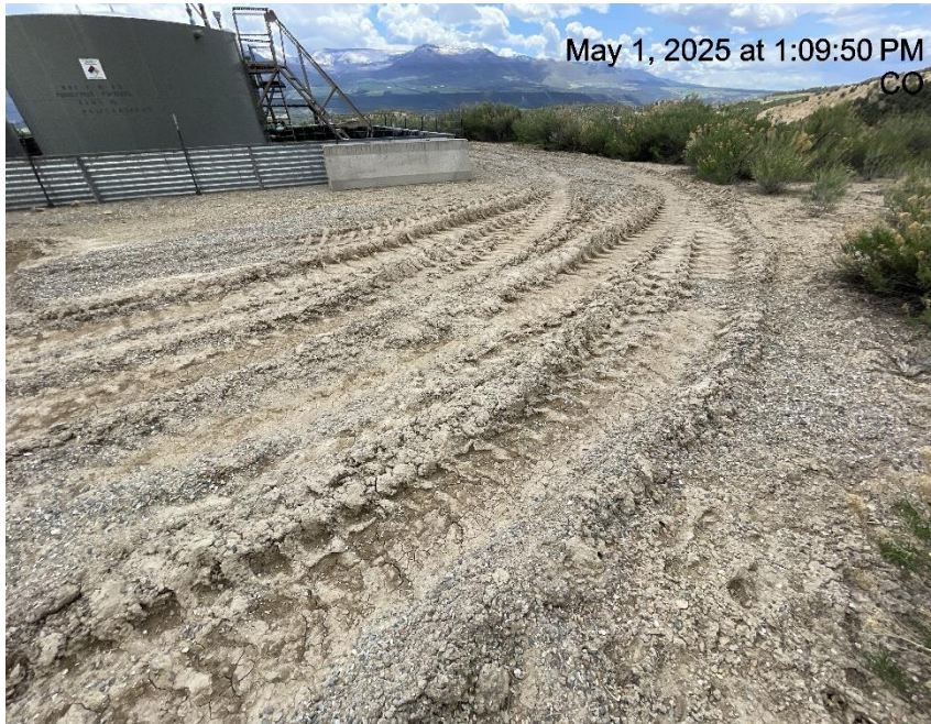
Photo # 7707 Lack of stabilization/compaction
