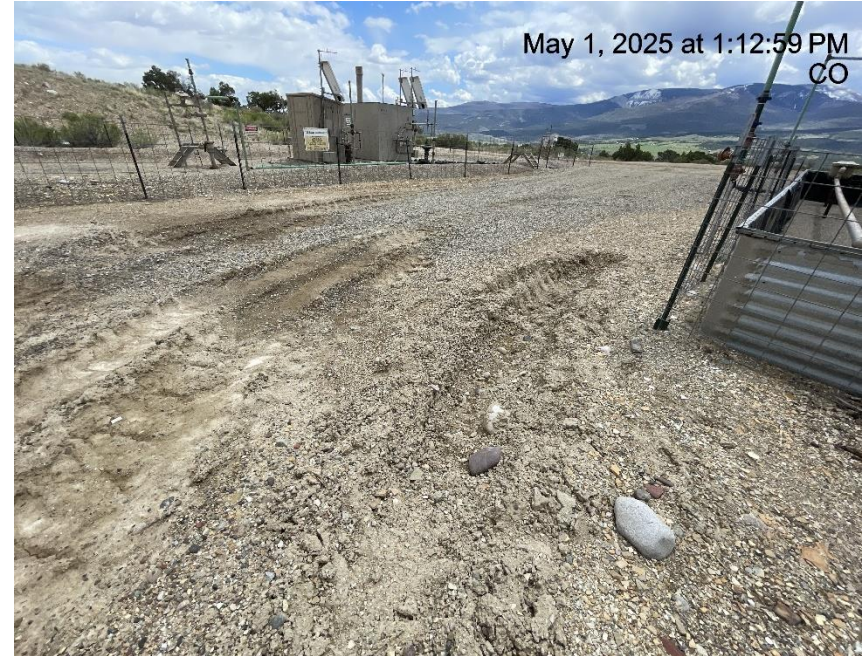
Photo # 7706 Lack of stabilization/compaction
