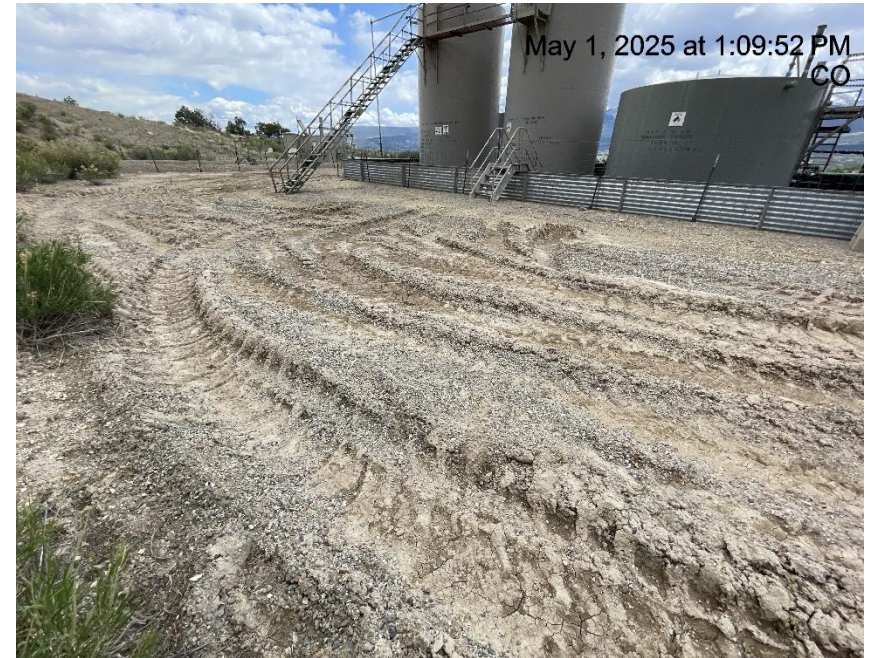
Photo # 7704 Lack of stabilization/compaction
