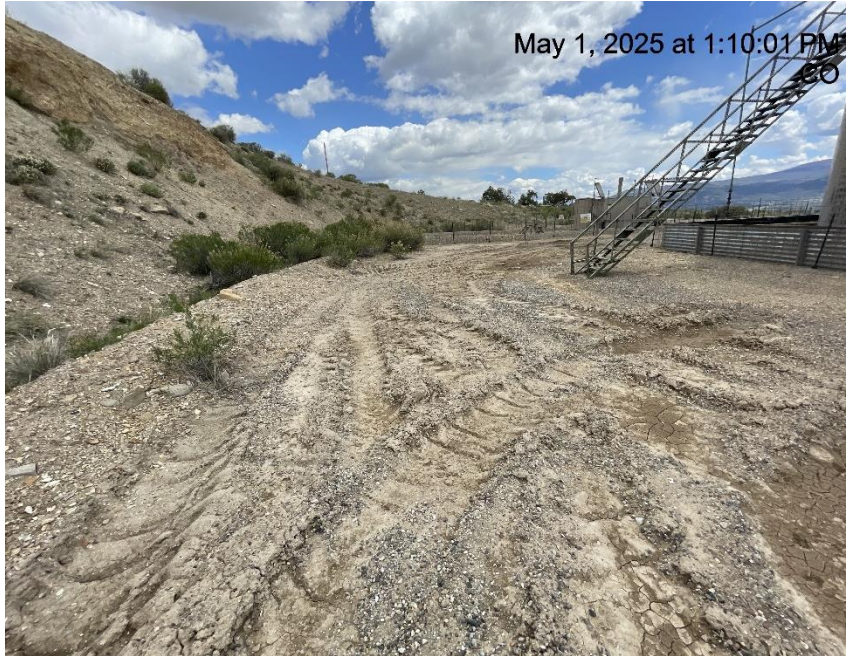
Photo # 7705 Lack of stabilization/compaction
