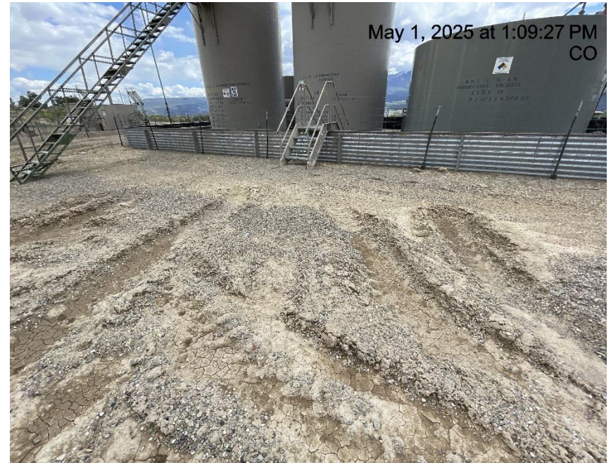
Photo # 7708 Lack of stabilization/compaction
