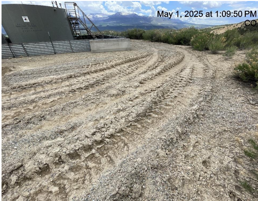
Photo # 7703 Lack of stabilization/compaction
