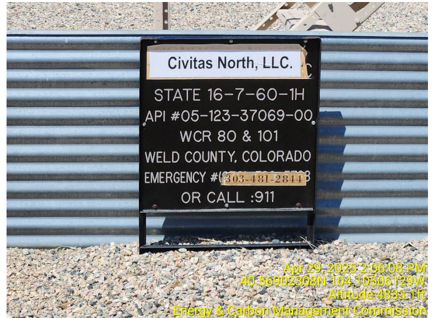
Photo 8 – Tank Battery Sign – Contact Number is Previous' Operarators
