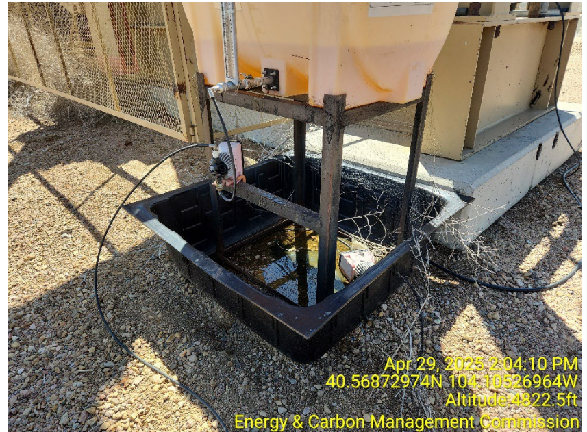
Photo 2 – Wildlife Netting in disrepair
