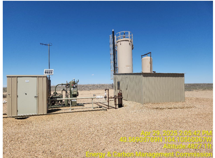
Photo 6 – Heater Treater, Gas Meter and VRU
