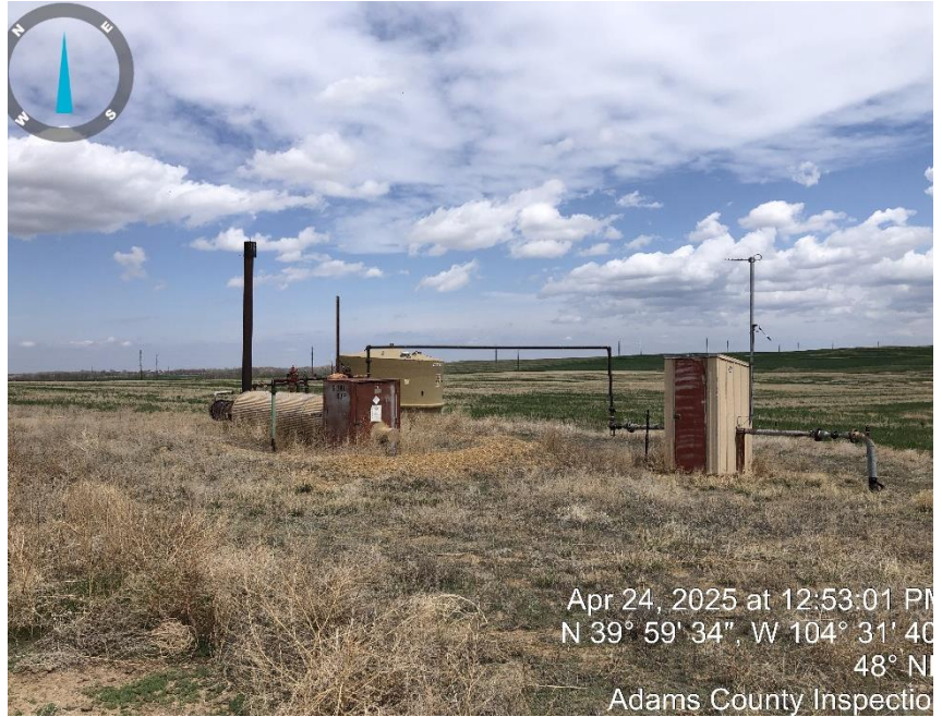
Photo #2 Separator & Meter (weeds)
