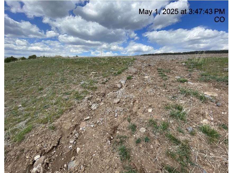
Photo # 7959 Failure to minimize erosion & the transport of sediment off location/insufficient BMP's (W/NW edge of location)
