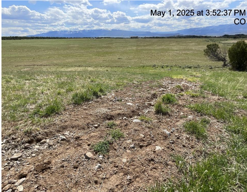
Photo # 7960 Failure to minimize erosion & the transport of sediment off location/insufficient BMP's (W/NW edge of location)
