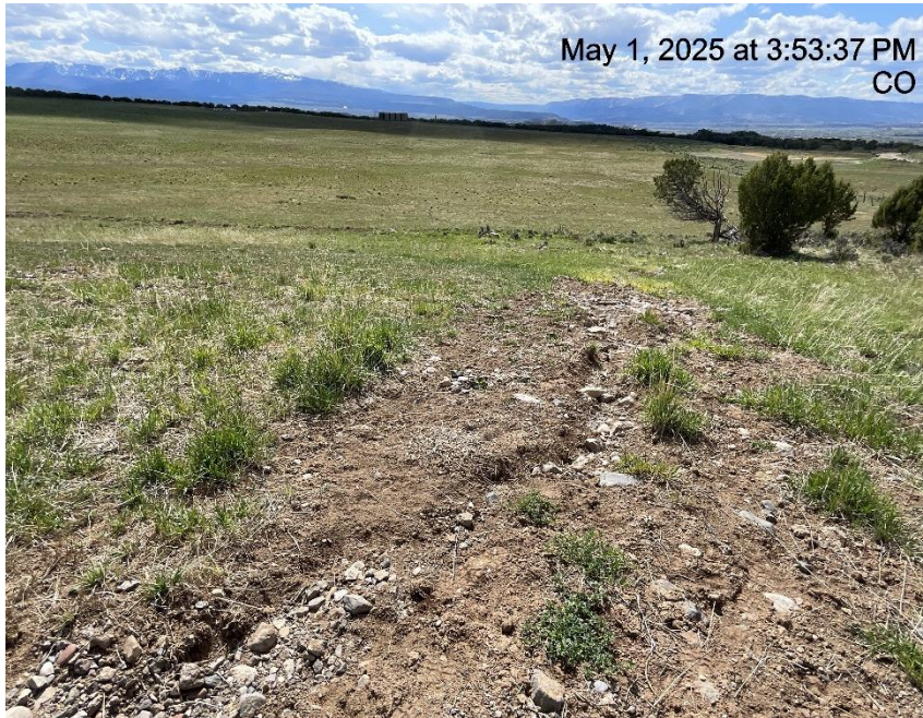
Photo # 7962 Failure to minimize erosion & the transport of sediment off location/insufficient BMP's (W/NW edge of location)
