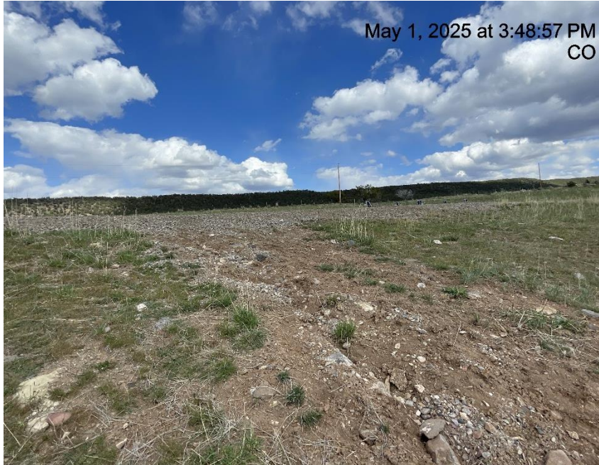
Photo # 7958 Failure to minimize erosion & the transport of sediment off location/insufficient BMP's (W/NW edge of location)
