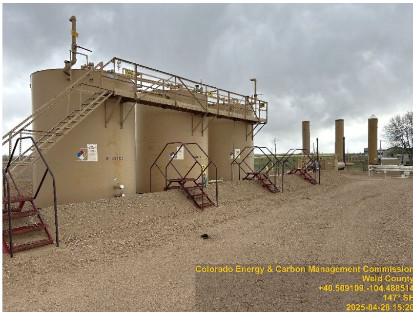
Photo #3 Foss 6-32, 6-31 Battery site Inactive | Shut-down Equipment documented: Fac. ID 487904 Formerly served: Foss 6-33, 6.34, 6-35 Plugged & Abandoned | PA
