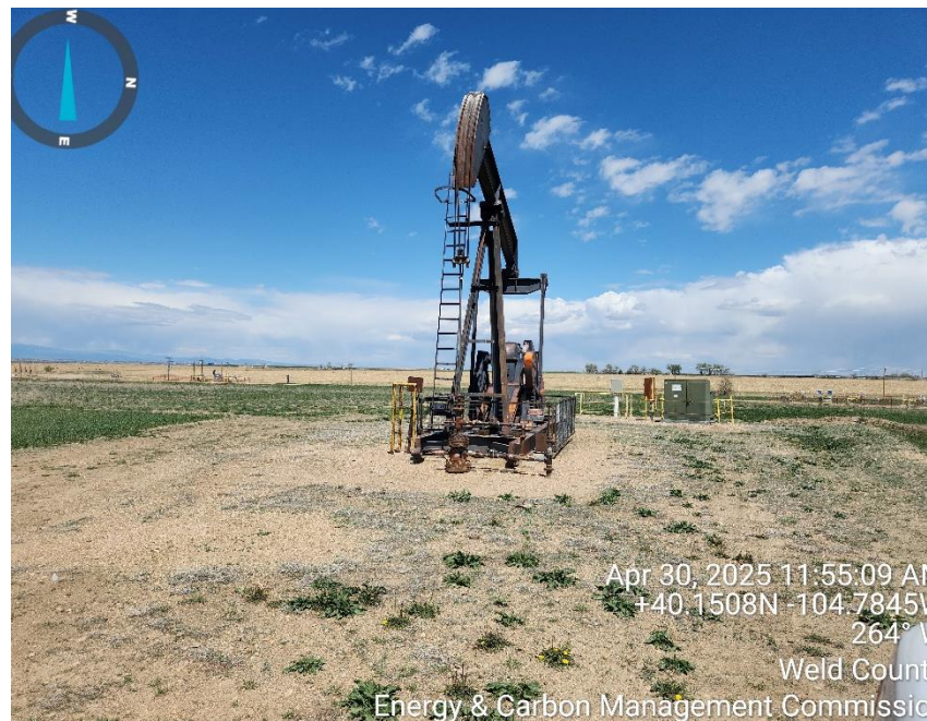
Photo 2 well head and equipment
