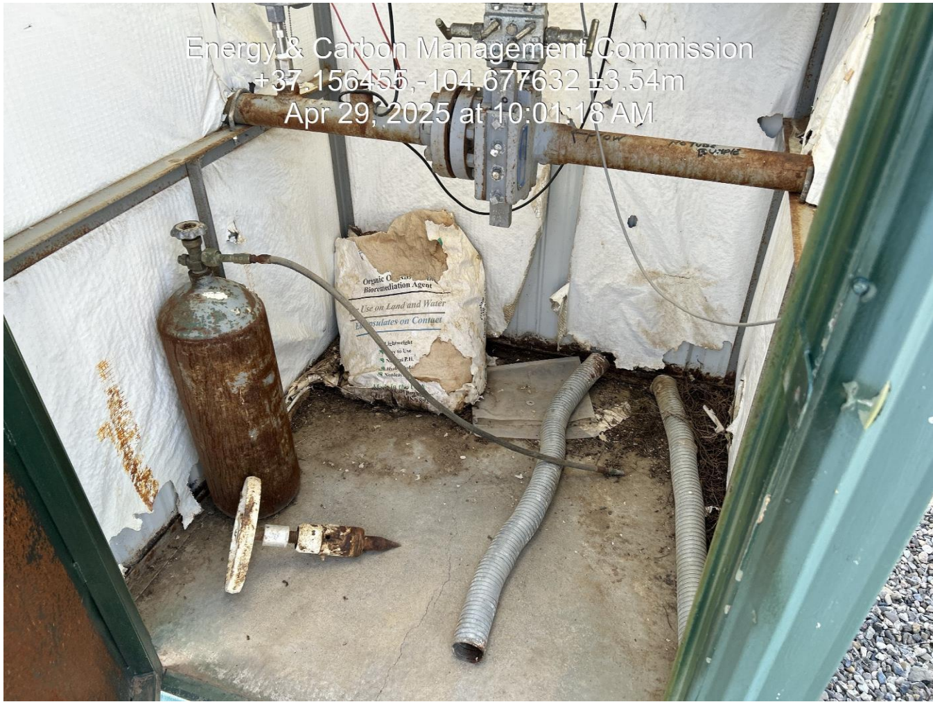
PHOTO 4: Trash in meter house needs to be removed
