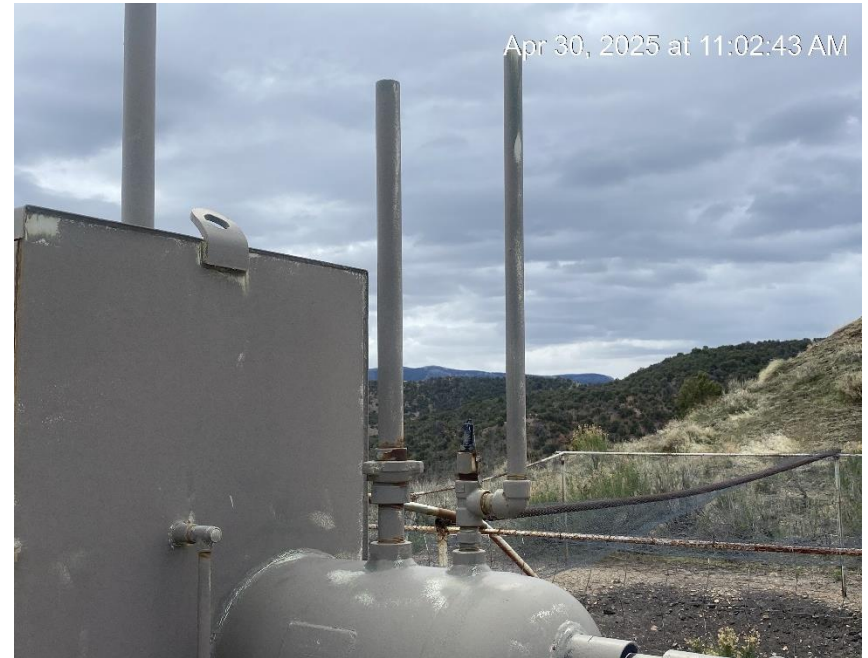
Unprotected relief vent risers
