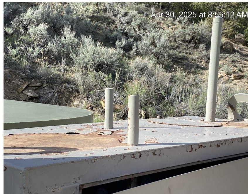
Unprotected vent risers
