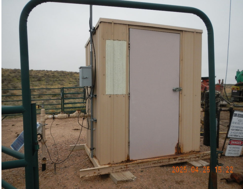
3. View of Gas Meter Shed at location.
