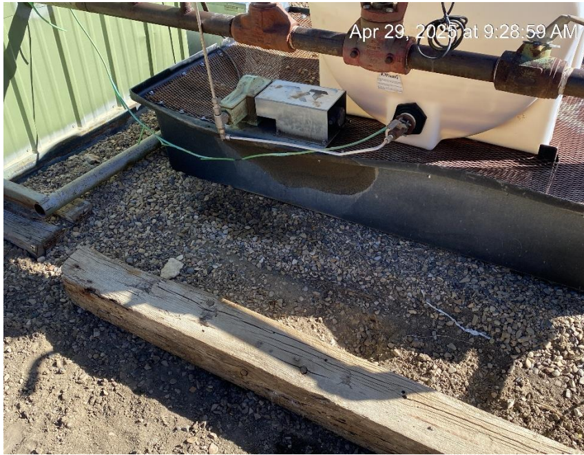
Leaking equipment and stained soil
