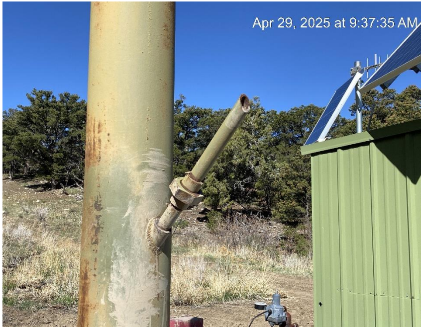
Riser cap required
