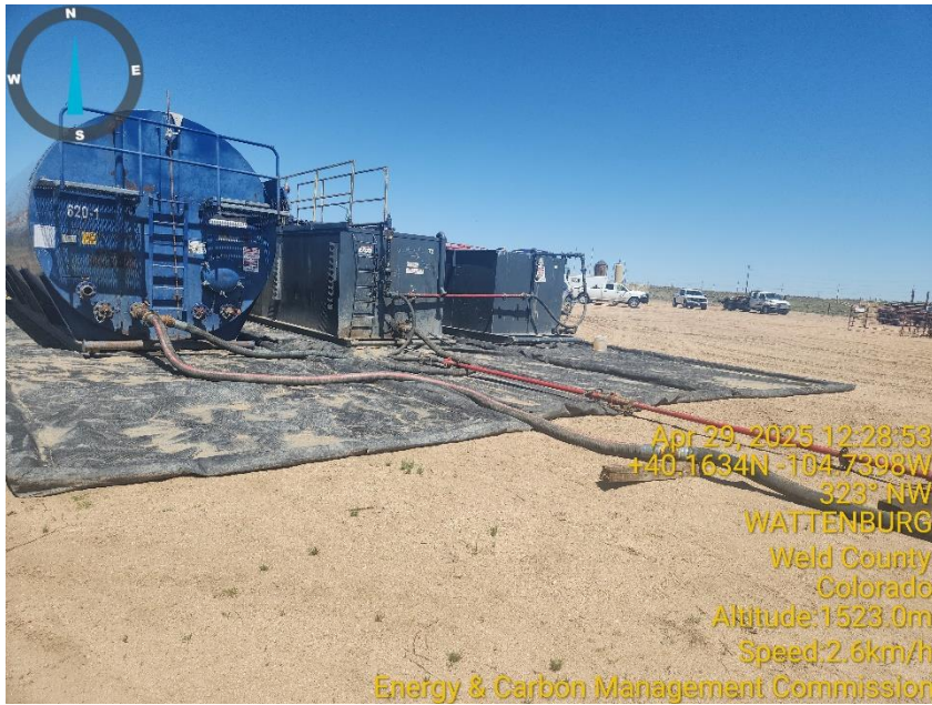
Photo 5 Fresh water & circulation tanks.
