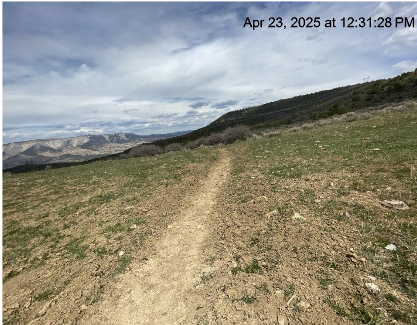
Photo # 4921 Ditch lacks any BMP's (N/NE area of location)
