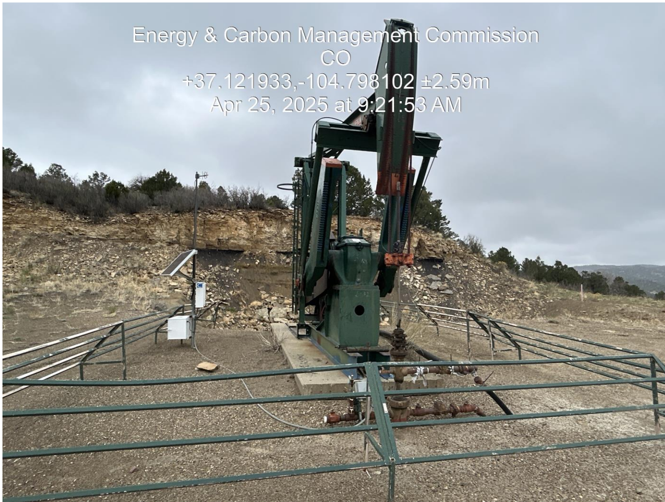
PHOTO 3: WELLHEAD AND EQUIPMENT
