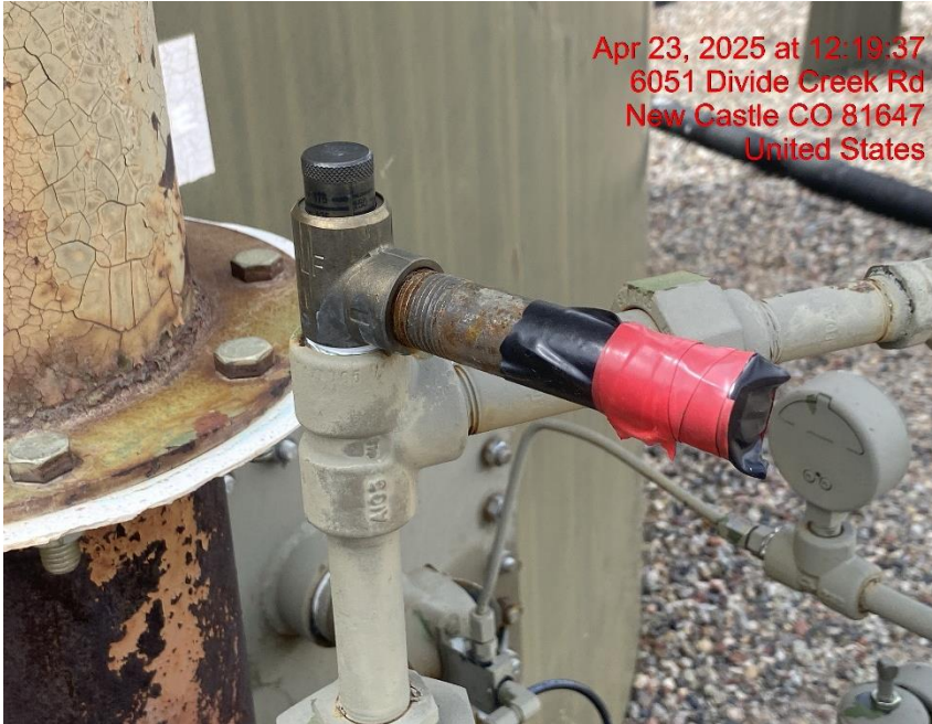
PRV Terminates in Unsafe Manner – Photo #08384
