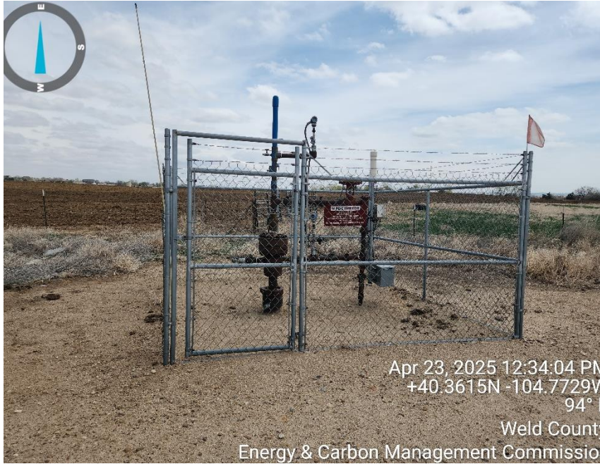
Photo 1 well head and equipment
