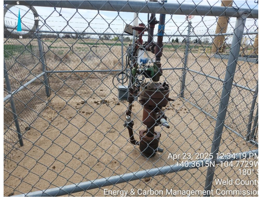
Photo 2 well head and equipment
