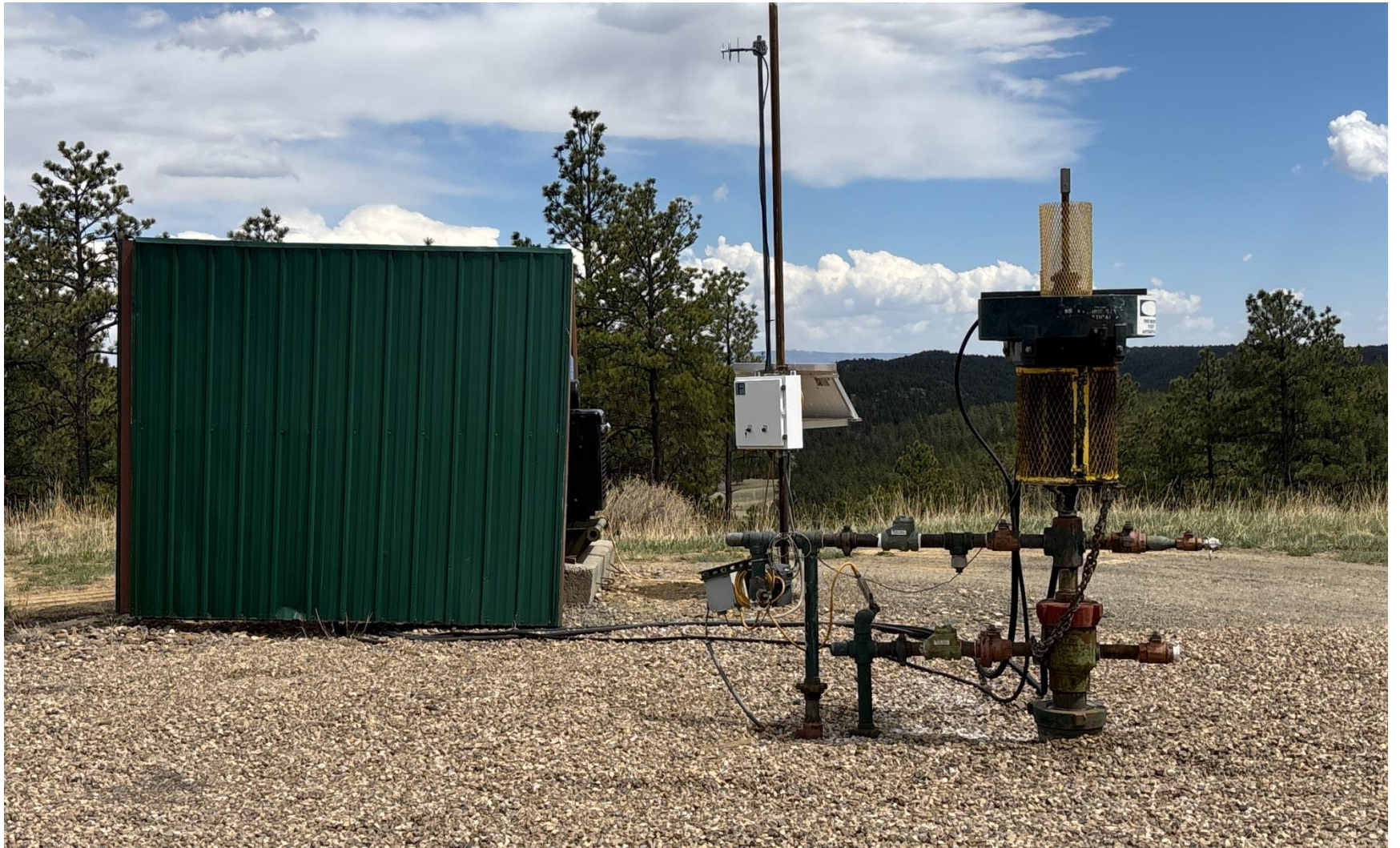
PHOTO 3: WELLHEAD AND EQUIPMENT.
