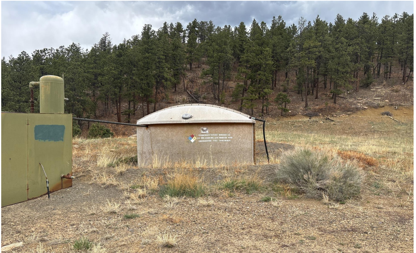
PHOTO 4: PRODUCED WATER TANK BATTERY/ WEEDS ON AND INSIDE BERMS. ALL VEGETATION MUST BE REMOVED INCLUDING ROOT STRUCTURED ON AND INSIDE ALL TANK BATTERY BERMS.
