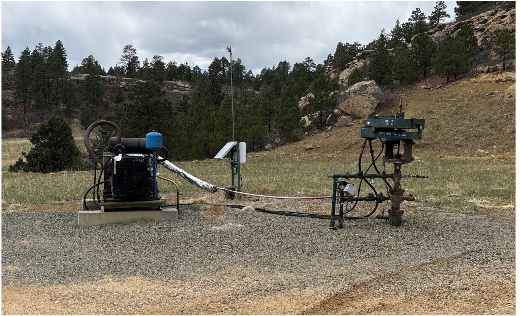
PHOTO 3: WELLHEAD AND EQUIPMENT.
