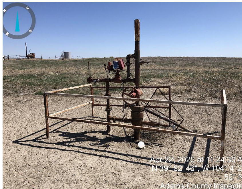
Photo #3 Well head.
