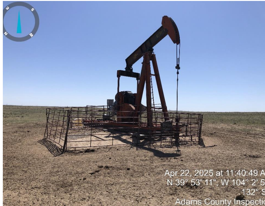
Photo # 3 Pump jack.
