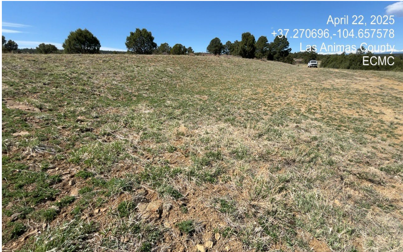
Photo 5. Facing west along the cut slope which is stabilized with perennial vegetation.
