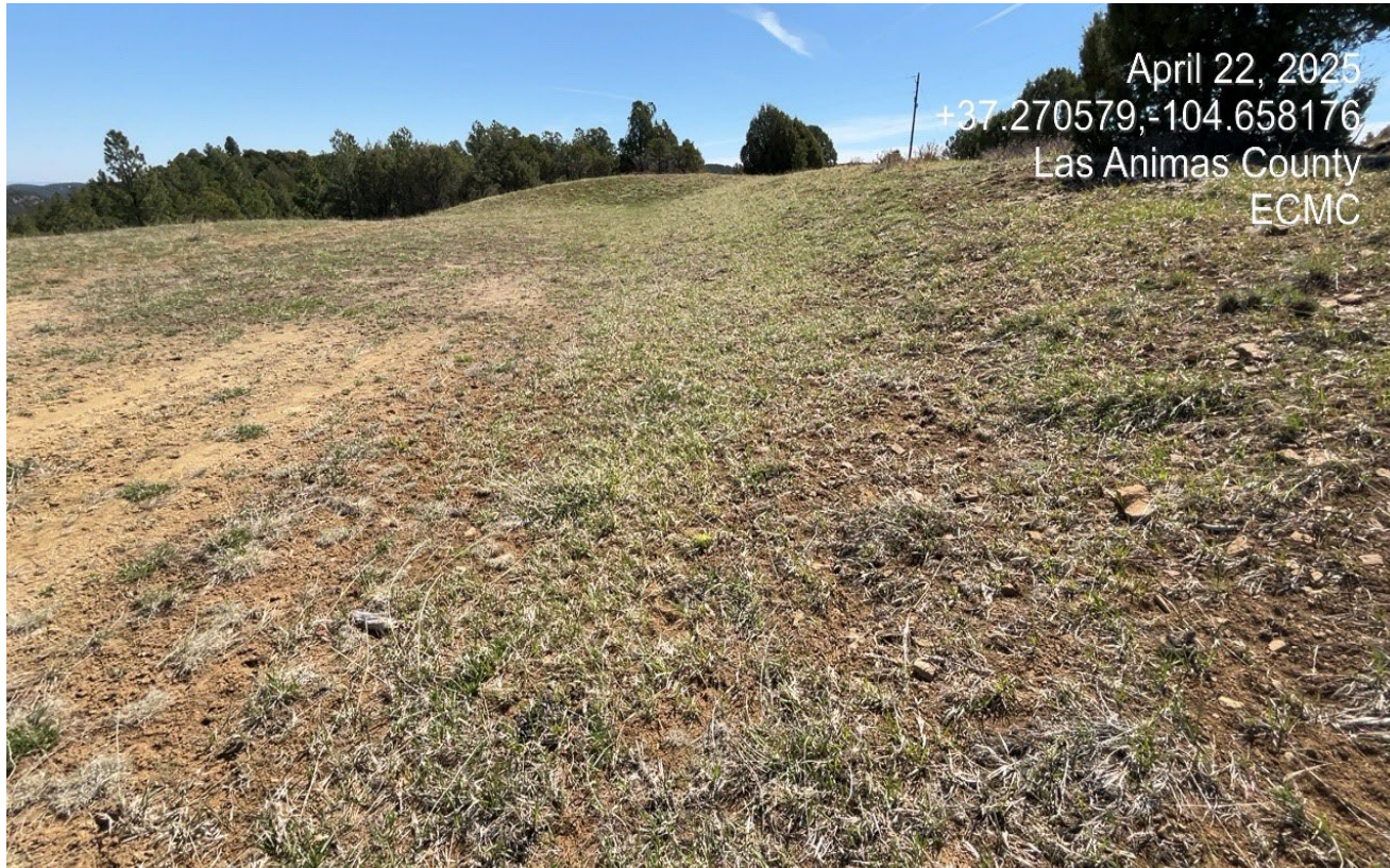
Photo 6. Facing east along the cut slope which is stabilized with perennial vegetation.
