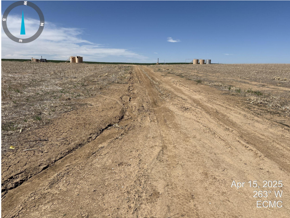
Photo 1. Looking west down the access road. Road is rutted resulting in widening of the road.
