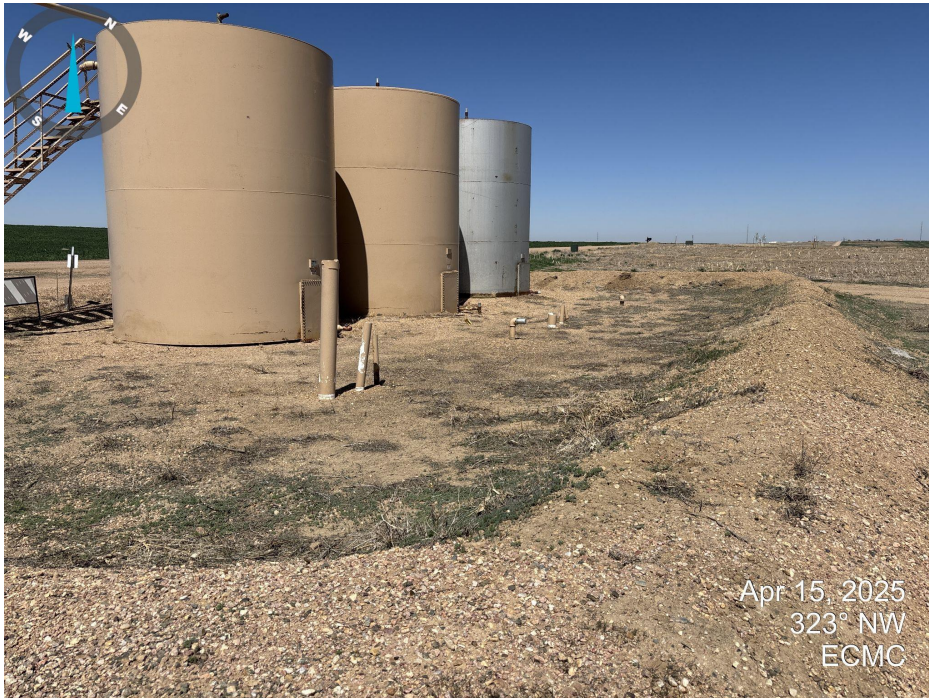
Photo 11. Looking at the east side of the tank battery. Weeds have been mowed on location. Bird protectors have not been installed on open pipes.
