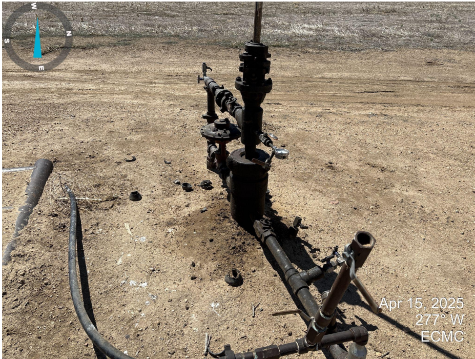
Photo 7. Southern side of wellhead. Wellhead does not appear to have active leaks. It appears that some stained soil was removed.
