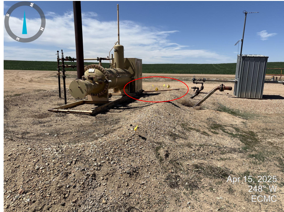
Photo 10. Looking at the north side of separator. Pipe remains at the separator (red circle).
