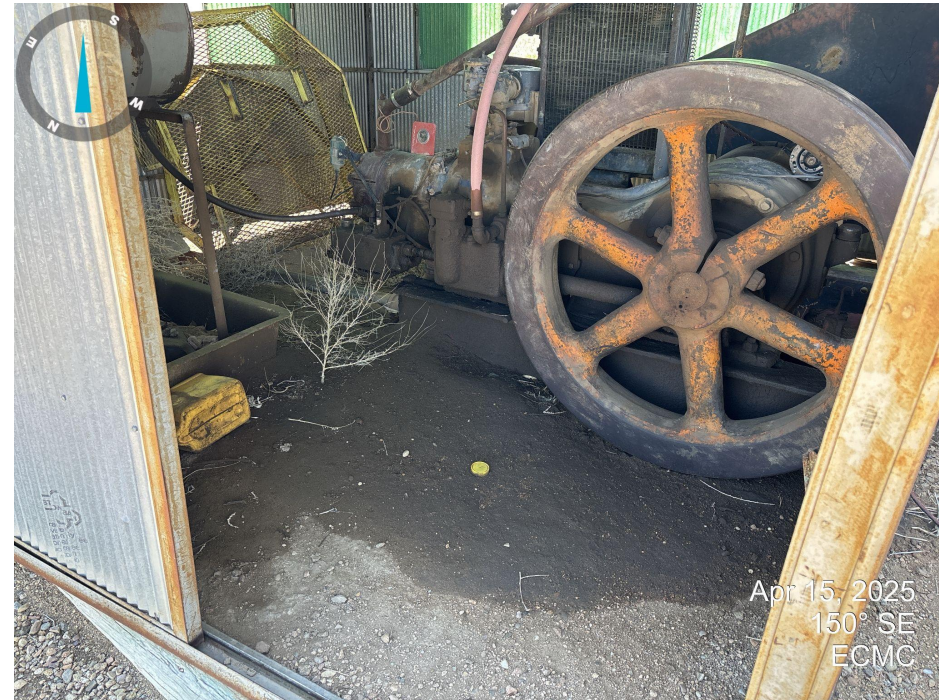
Photo 4. Inside the engine shed. Stained soil is present around the engine. The engine was not running at time of inspection. Engine guard is not installed.
