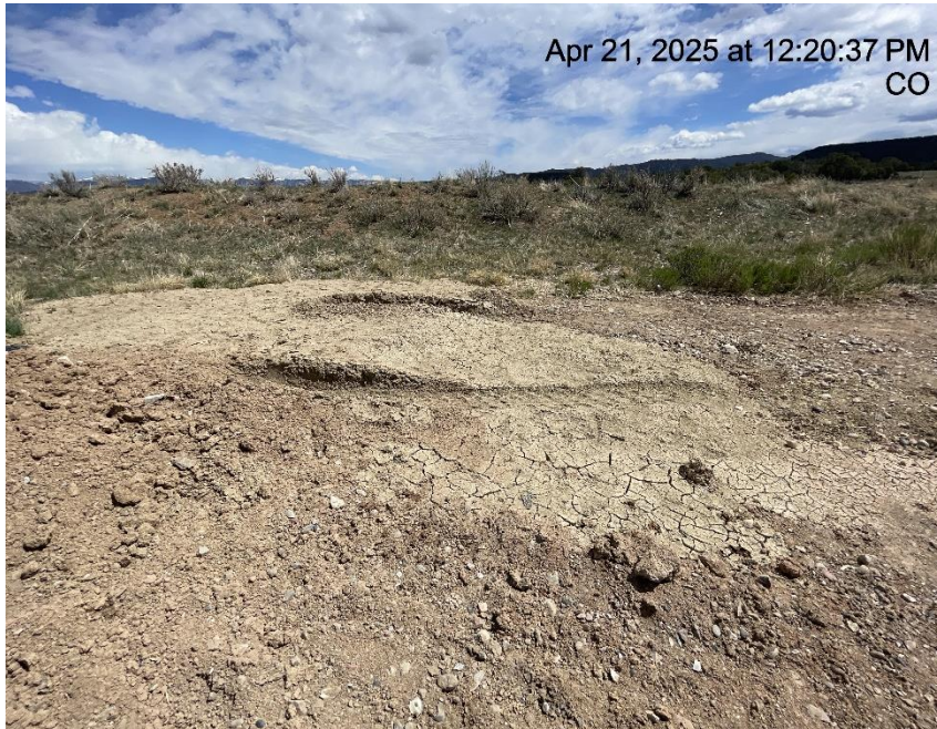
Photo # 3598 Stockpiled soils with no BMP's/not in compliance with CECMC Stormwater rules
