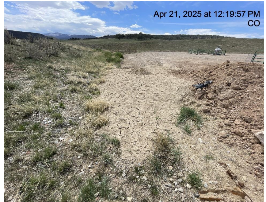
Photo # 3599 Stockpiled soils with no BMP's/not in compliance with CECMC Stormwater rules
