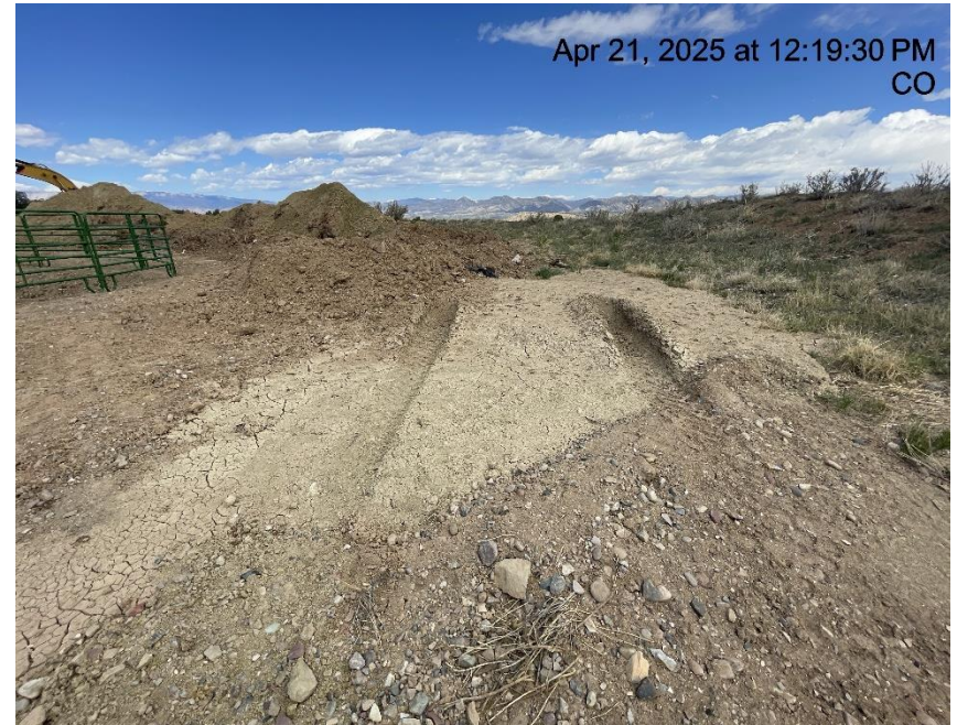
Photo # 3597 Stockpiled soils with no BMP's/not in compliance with CECMC Stormwater rules
