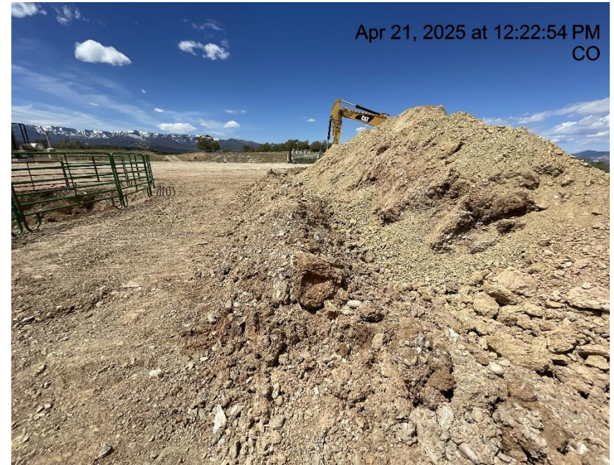
Photo # 3593 Insufficient BMP's around stockpiled soils/BMP not constructed in accordance with good engineering practices/not in compliance with CECMC Stormwater rules
