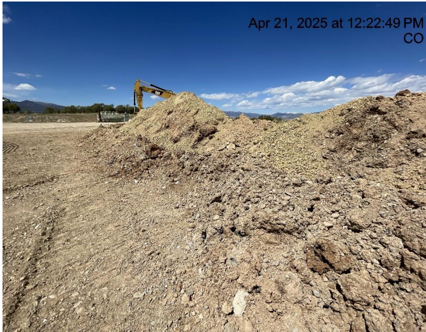
Photo # 3592 Insufficient BMP's around stockpiled soils/BMP not constructed in accordance with good engineering practices/not in compliance with CECMC Stormwater rules
