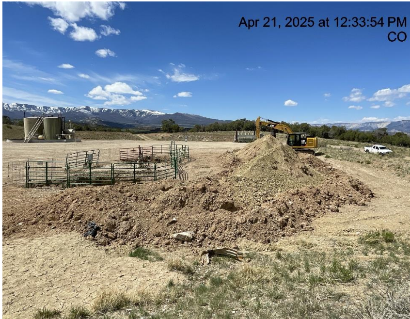
Photo # 3580 Stockpiled soils with insufficient BMP's
