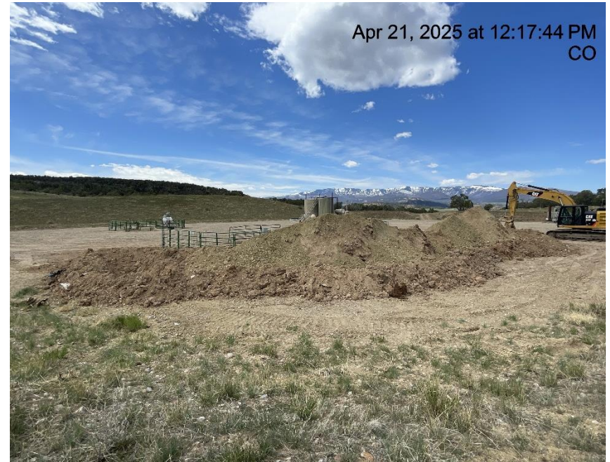
Photo # 3579 Stockpiled soils with insufficient BMP's
