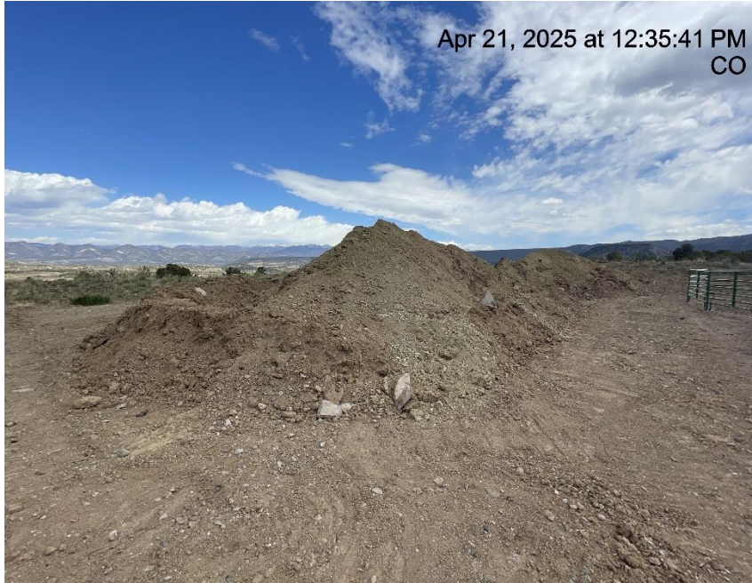
Photo # 3582 Stockpiled soils with insufficient BMP's
