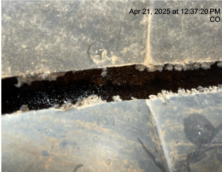
Photo # 3576 Failure to maintain chemical BMP - Chemical tank containment full of fluid/BMP insufficient to contain possible spill
