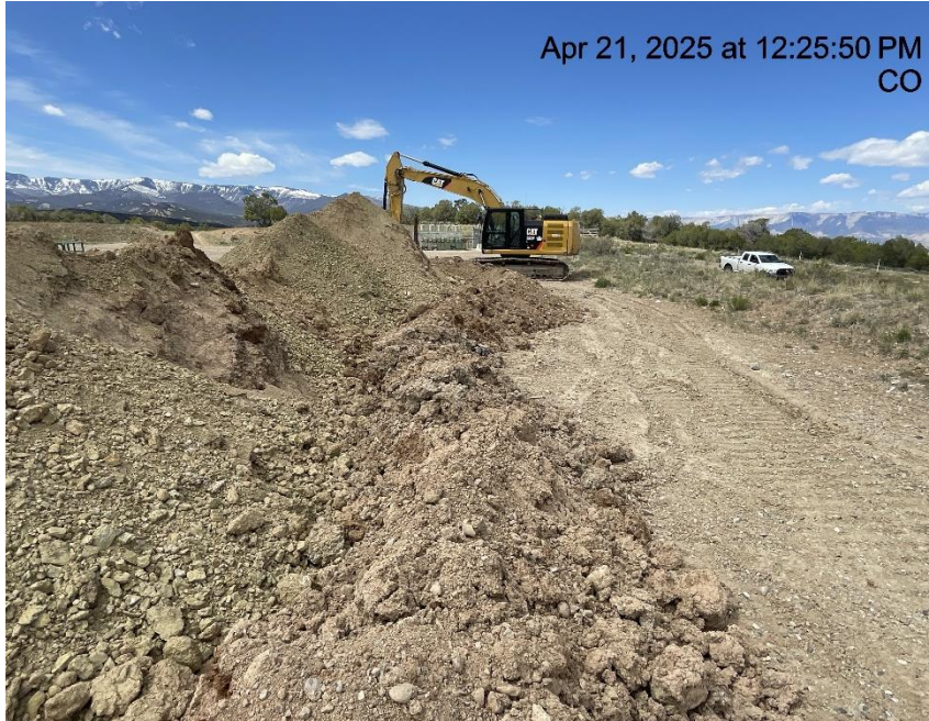
Photo # 3584 Insufficient BMP's around stockpiled soils/BMP not constructed in accordance with good engineering practices/not in compliance with CECMC Stormwater rules
