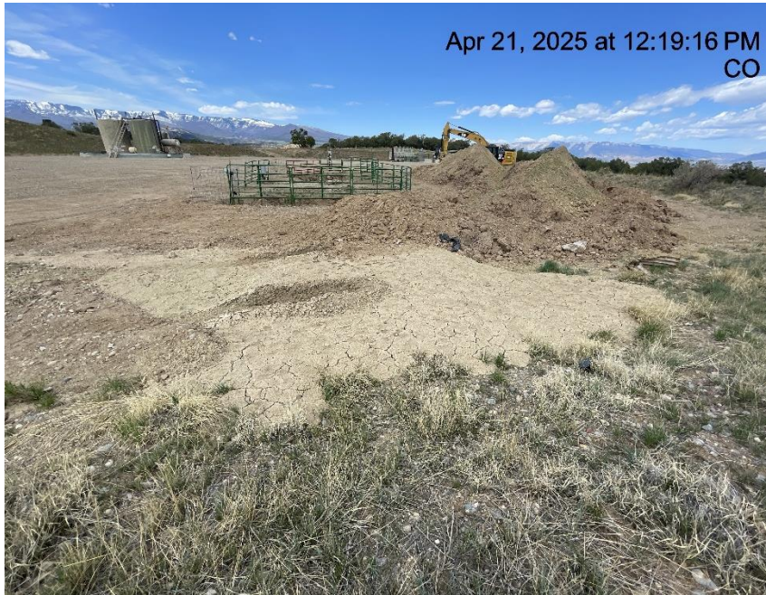
Photo # 3594 Stockpiled soils with no BMP's/not in compliance with CECMC Stormwater rules
