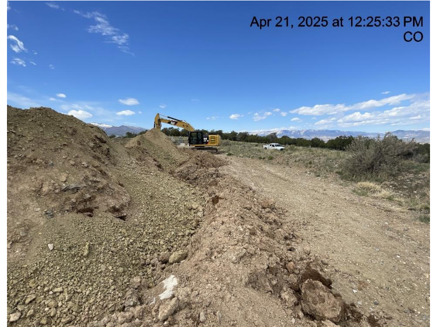
Photo # 3585 Insufficient BMP's around stockpiled soils/BMP not constructed in accordance with good engineering practices/not in compliance with CECMC Stormwater rules
