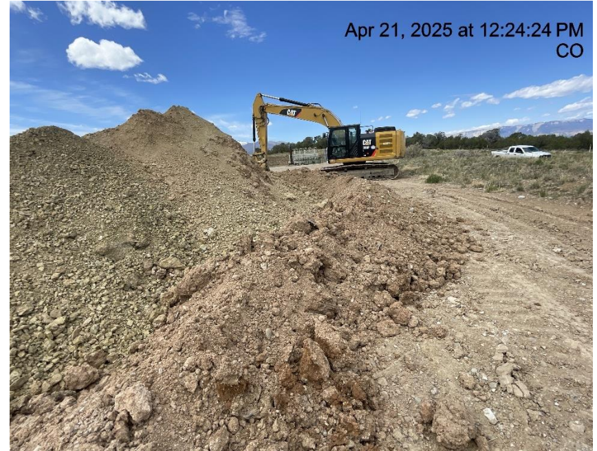
Photo # 3583 Insufficient BMP's around stockpiled soils/BMP not constructed in accordance with good engineering practices/not in compliance with CECMC Stormwater rules
