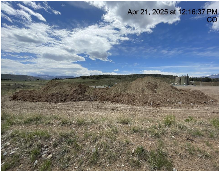
Photo # 3578 Stockpiled soils with insufficient BMP's
