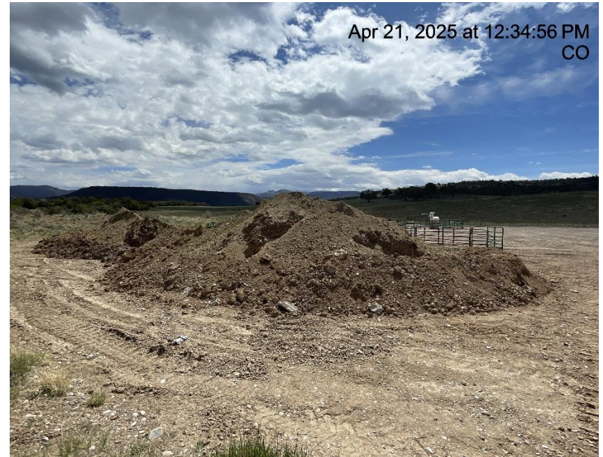
Photo # 3581 Stockpiled soils with insufficient BMP's
