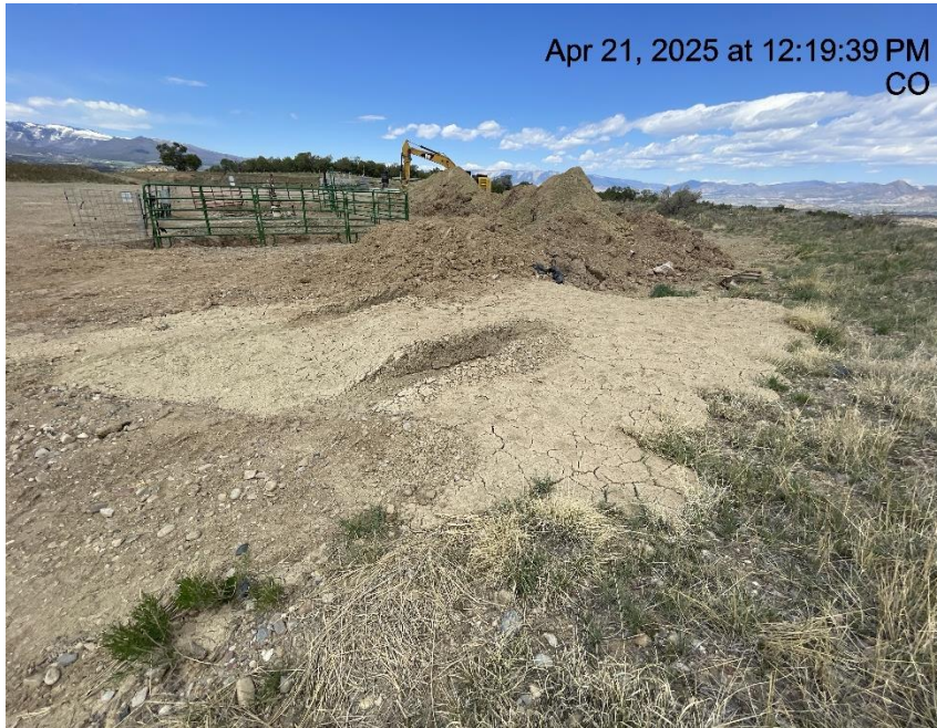
Photo # 3596 Stockpiled soils with no BMP's/not in compliance with CECMC Stormwater rules
