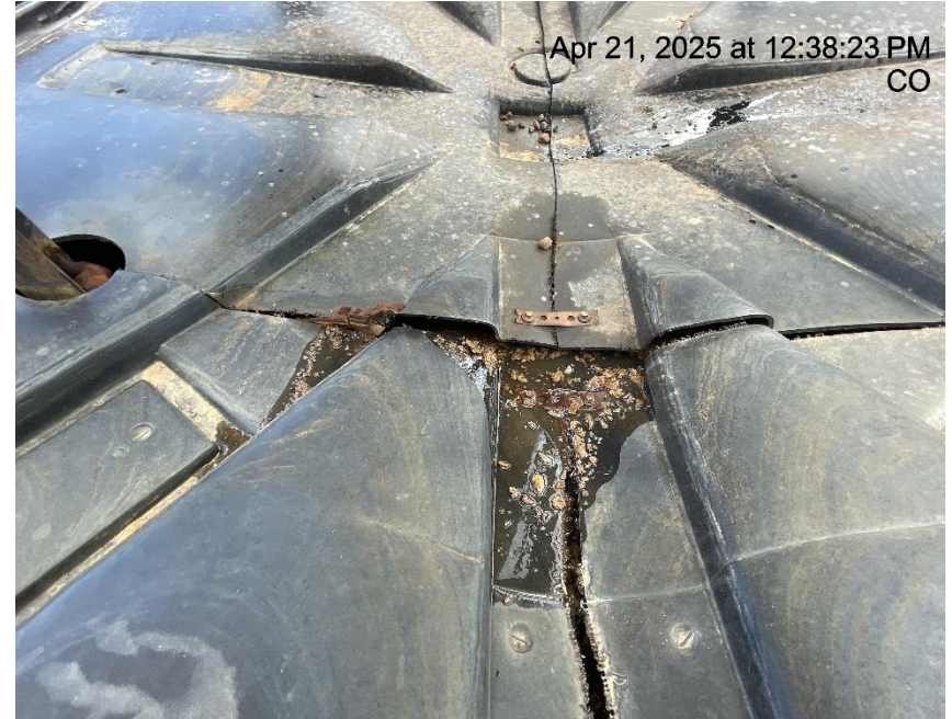
Photo # 3577 Failure to maintain chemical BMP - Chemical tank containment full of fluid/BMP insufficient to contain possible spill
