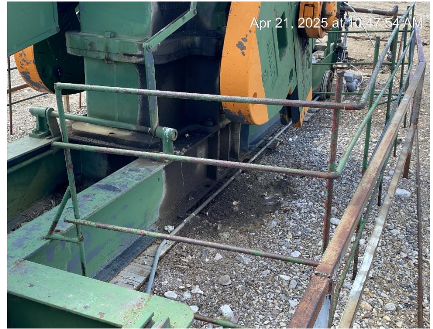
Leaking equipment with stained soil
