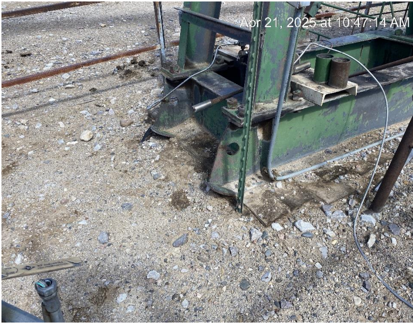
Debris. Stained soil.
