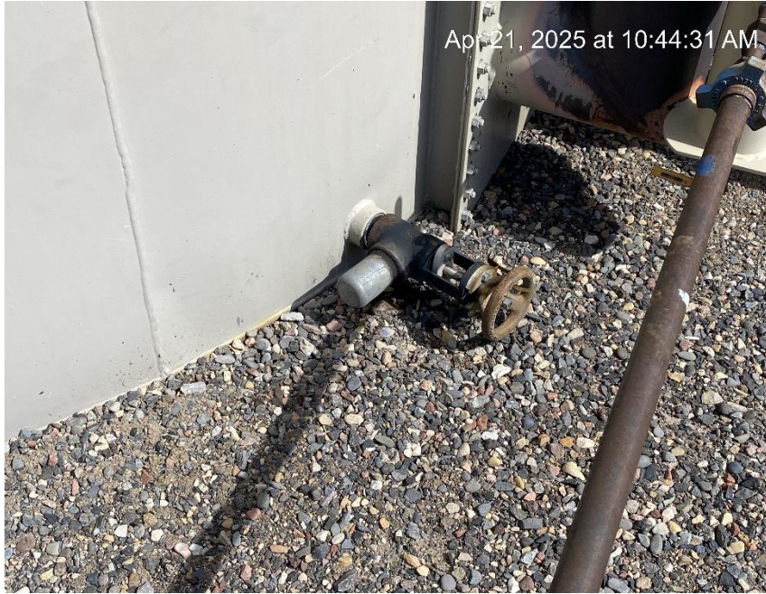
Stained soil below valve
