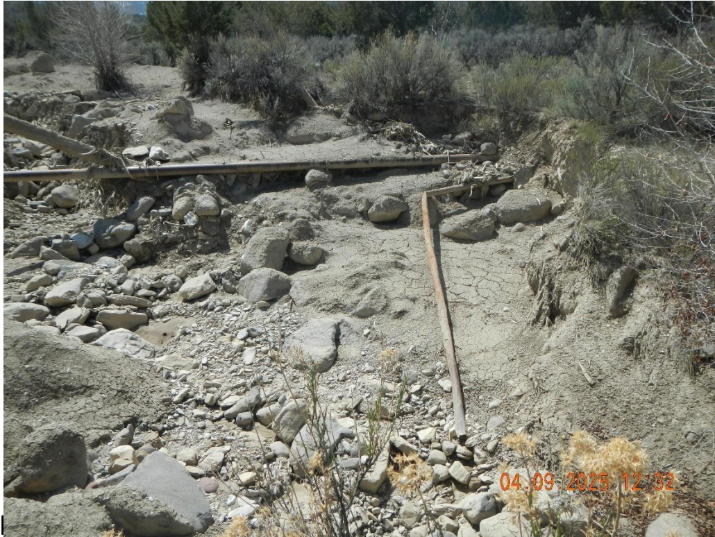
4" flowline open ended and bent. 8" pipe used to sleeve Mustangs flowline to Burns #9-35-6-94W well.
