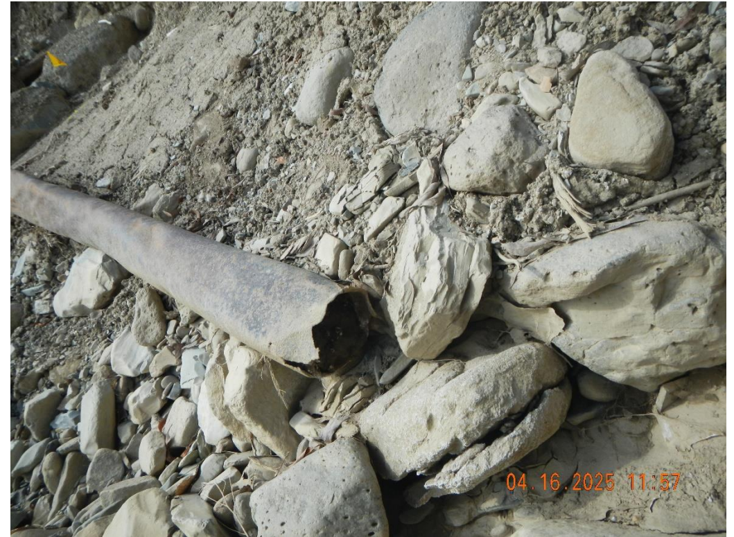
Photos from 4/16/2025 Open ended flowline
