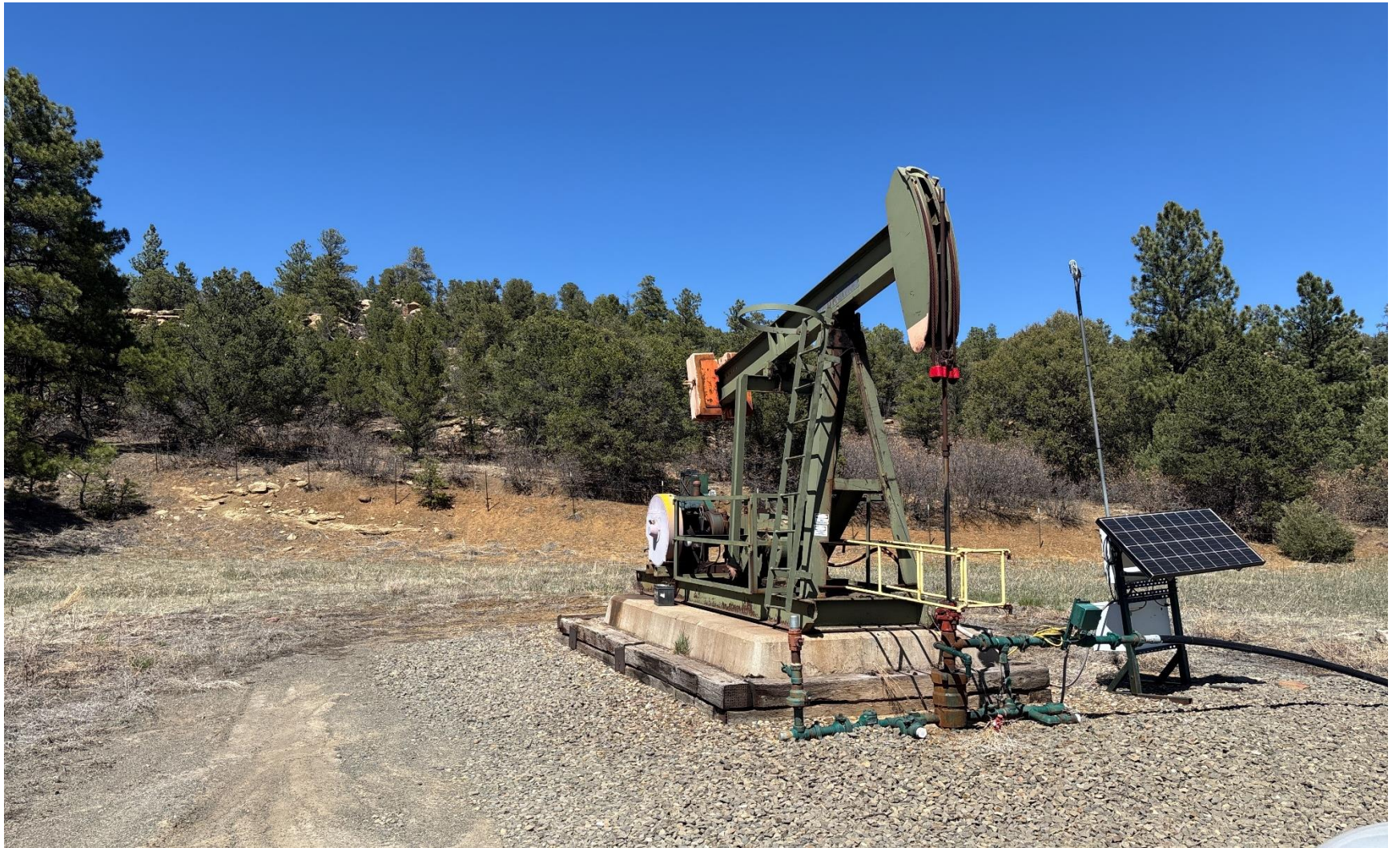
PHOTO 3: WELLHEAD AND EQUIPMENT.
