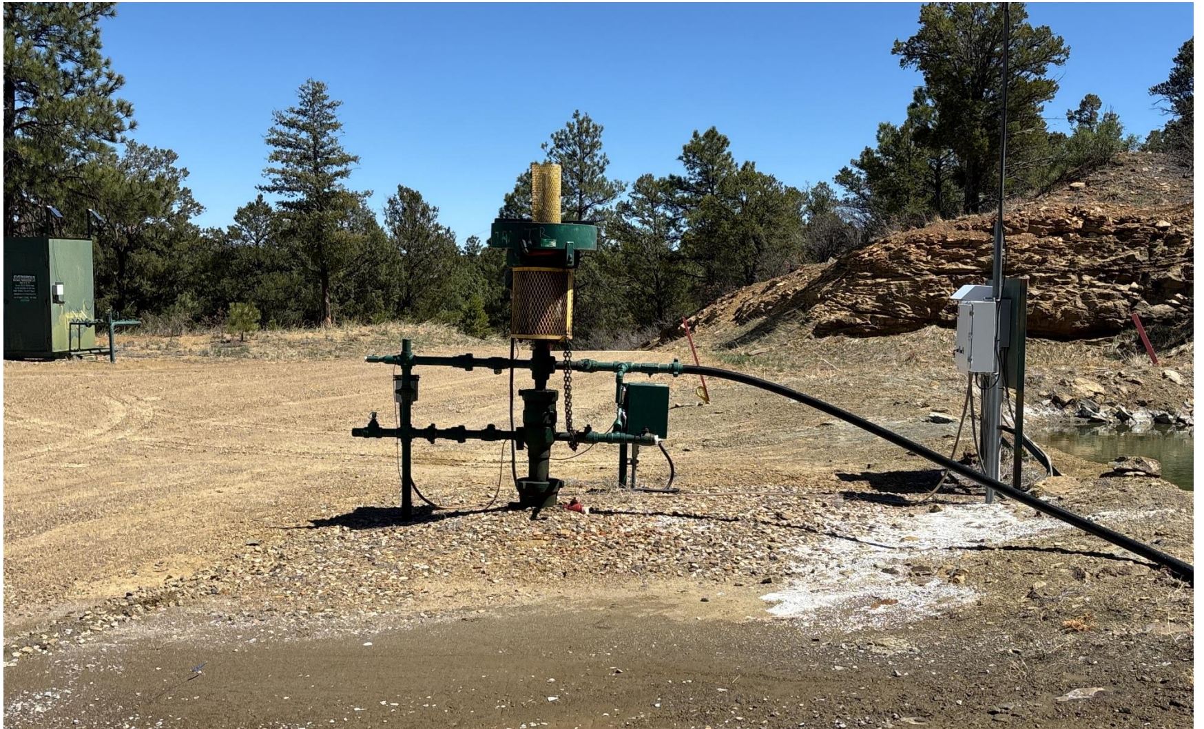
PHOTO 4: TR WELLHEAD AND EQUIPMENT.
