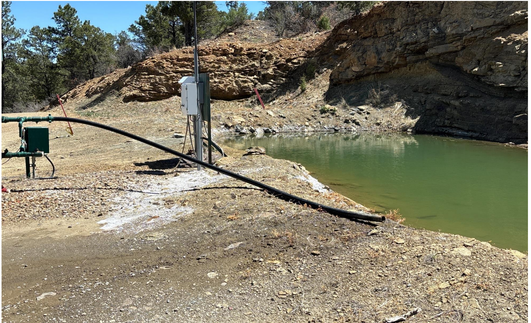
PHOTO 5: PRODUCED WATER LINE TO PIT IS ON THE PIT BERM AND SOME OF THE PRODUCED WATER IS FLOWING ONTO LOCATION. RE- POSITION FLOWLINE AND ANCHOR TO PREVENT ANY PRODUCED WATER TO FLOW ON LOCATION. CA DATE 4/18/2025.
