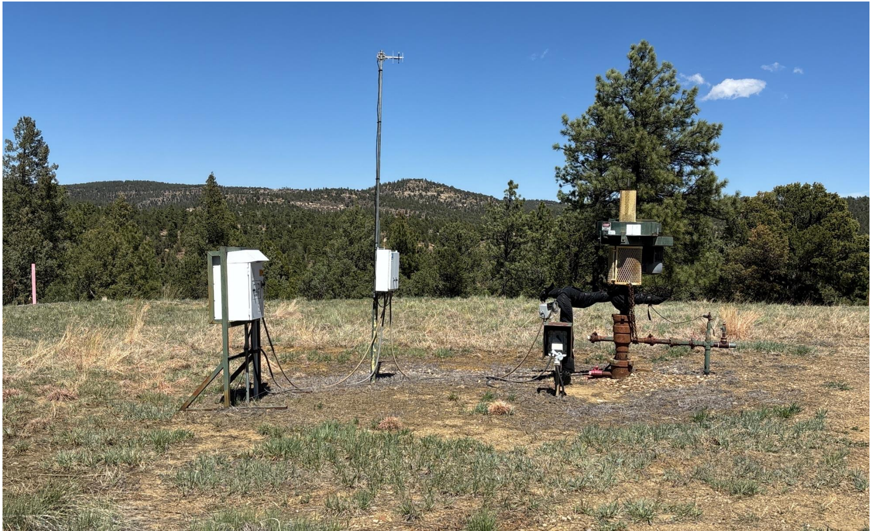
PHOTO 3: WELLHEAD AND EQUIPMENT.
