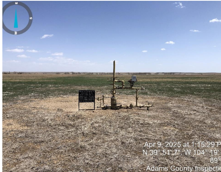
Photo #3 Well head.
