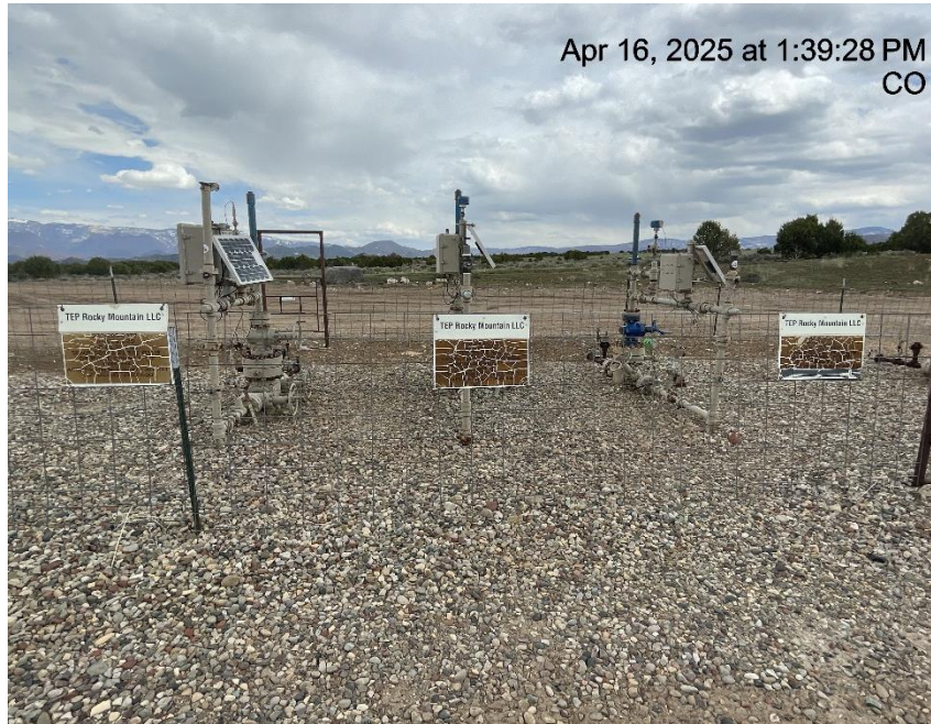
Photo # 2068 Multiple wellhead signs weathered & illegible /not in compliance with CECMC rules
