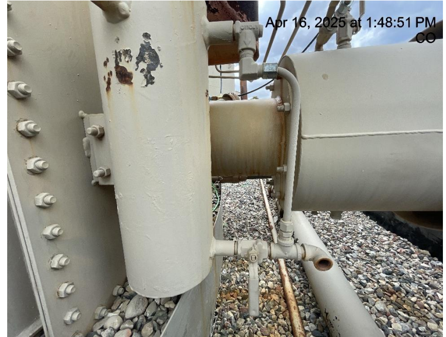
Photo # 2067 PRV vent line does not comply with CECMC pressure safety device rules or general safety rules
