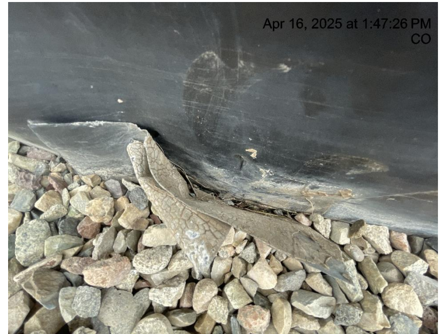
Photo # 2071 Hole in secondary containment liner/liner needs maintenance
