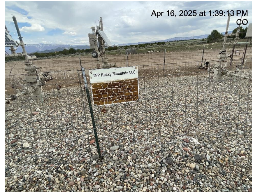
Photo # 2069 Wellhead sign weathered & illegible/not in compliance with CECMC rules
