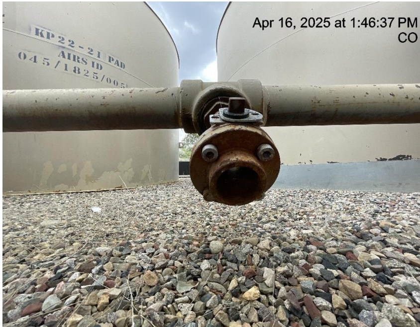
Photo # 2064 Open ended load line
