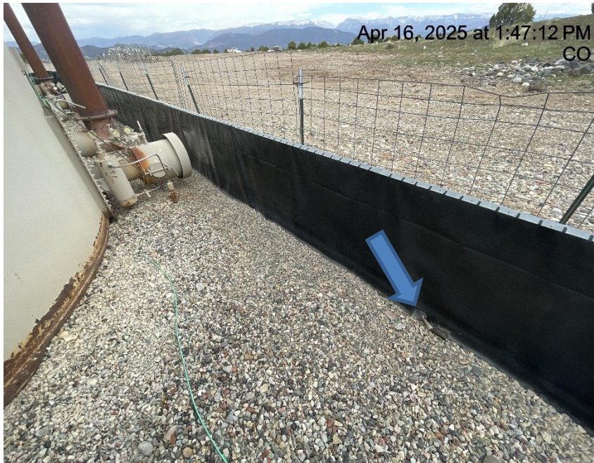
Photo # 2070 Hole in secondary containment liner/liner needs maintenance
