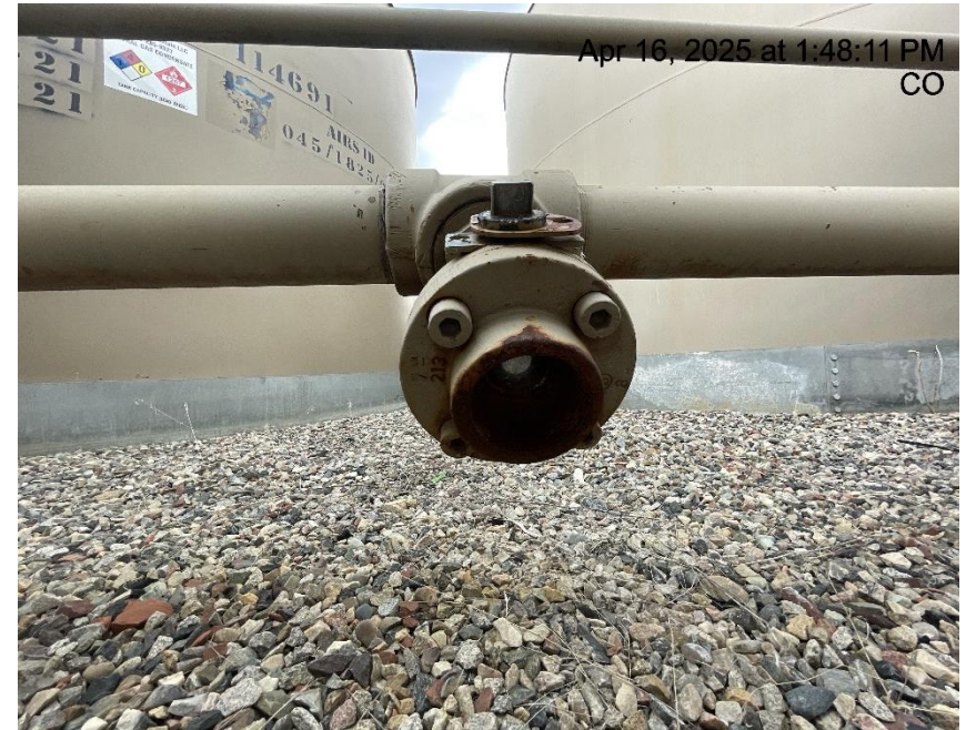
Photo # 2065 Open ended load line
