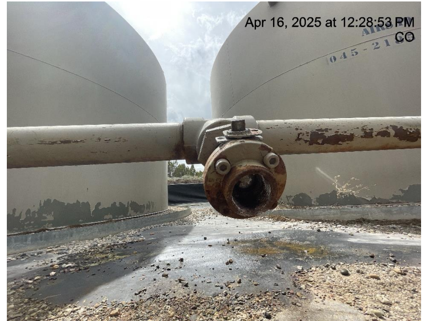
Photo # 1800 Open ended load line
