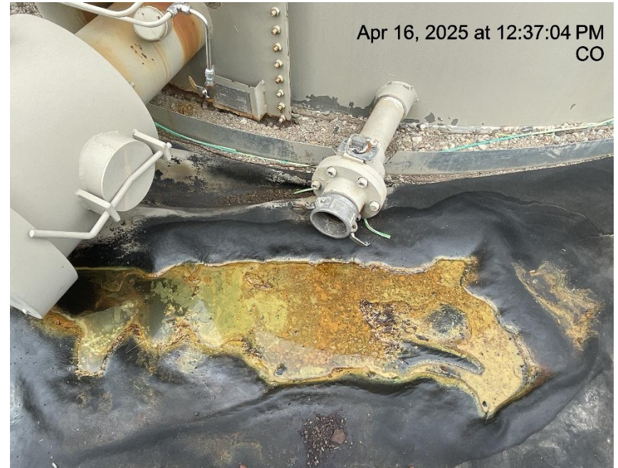
Photo # 1794 E & P waste in secondary containment
