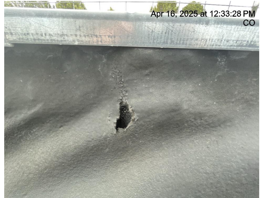
Photo # 1806 Hole in secondary containment liner/liner needs maintenance
