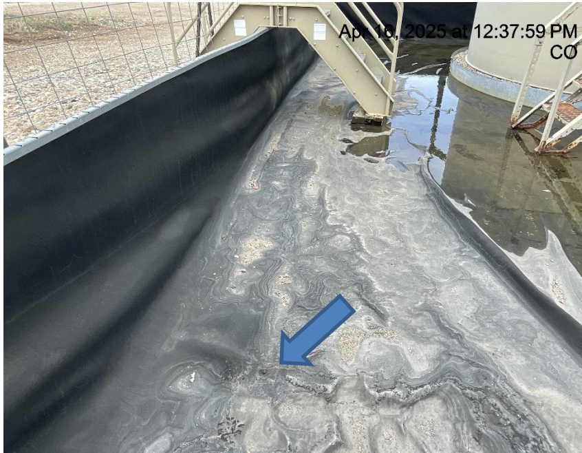
Photo # 1803 Hole in secondary containment liner/liner needs maintenance
