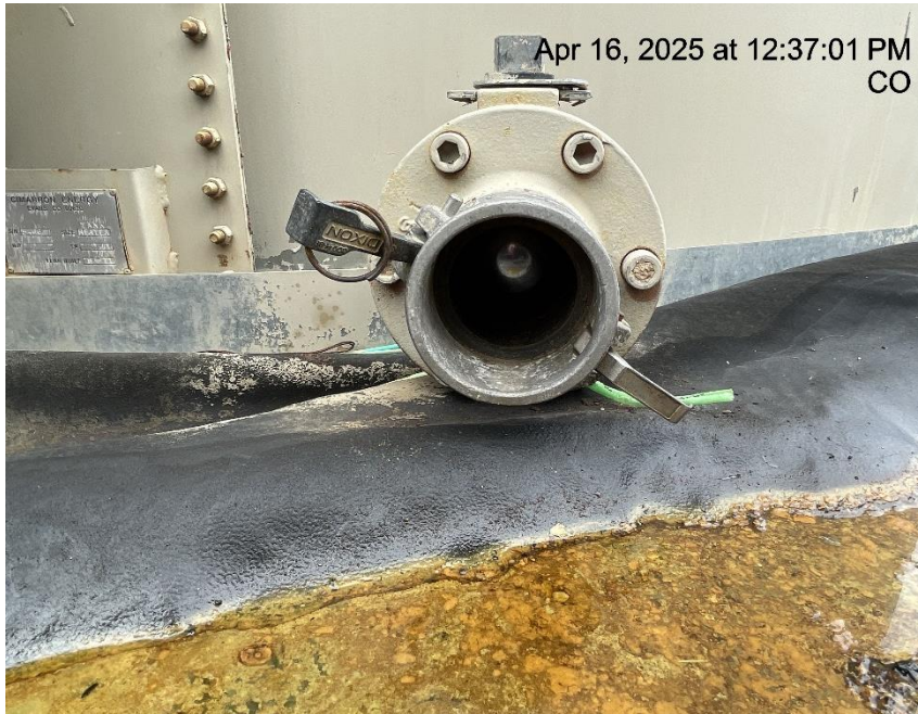
Photo # 1795 Open ended load line
