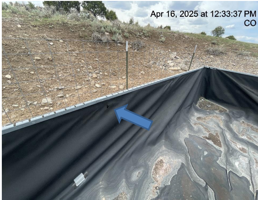
Photo # 1805 Hole in secondary containment liner/liner needs maintenance
