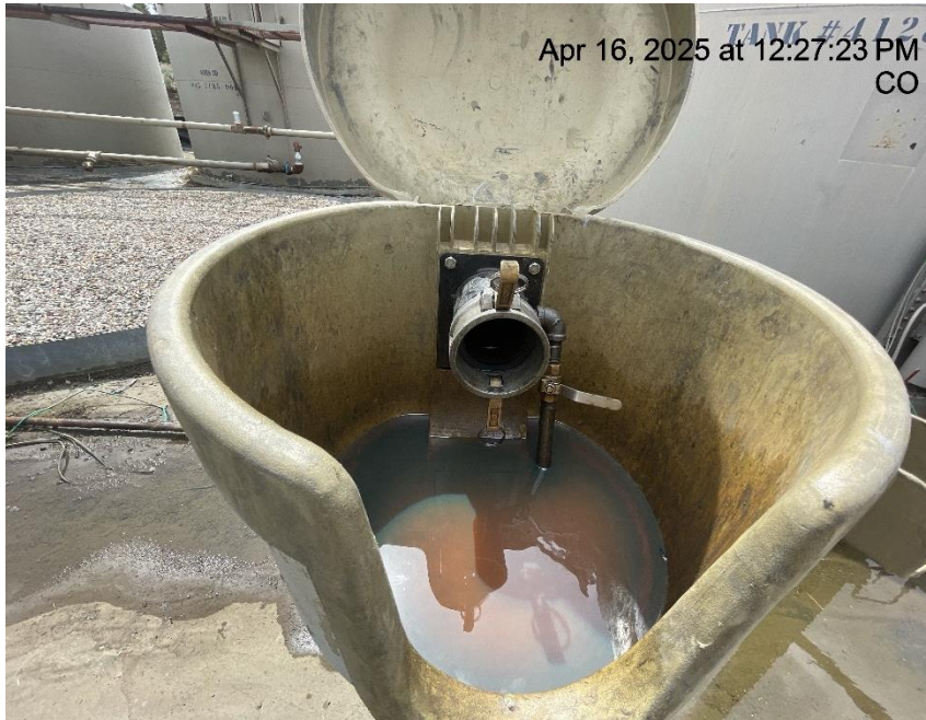
Photo # 1801 Open ended load line
