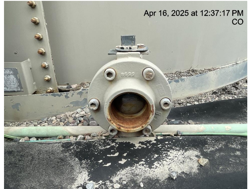
Photo # 1796 Open ended load line
