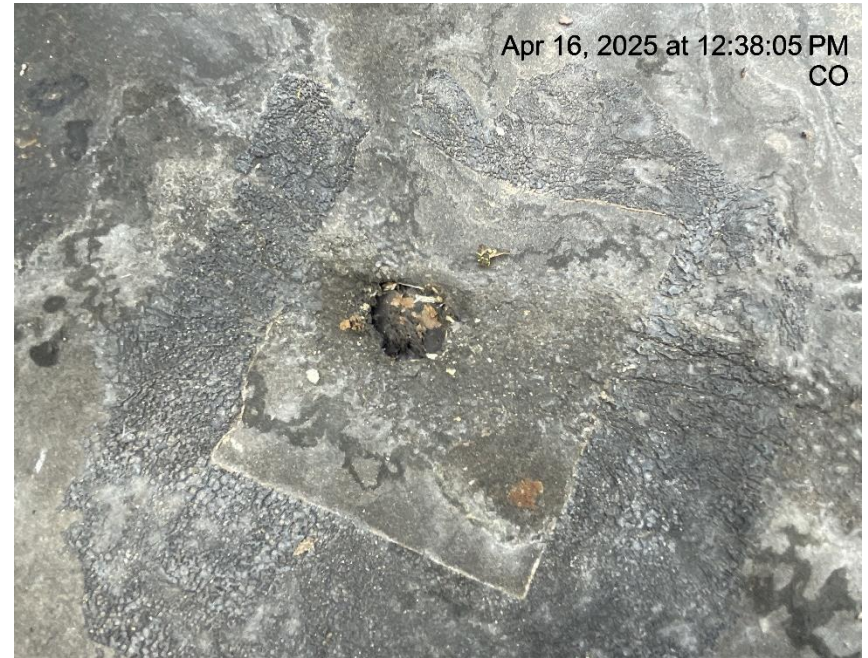
Photo # 1804 Hole in secondary containment liner/liner needs maintenance
