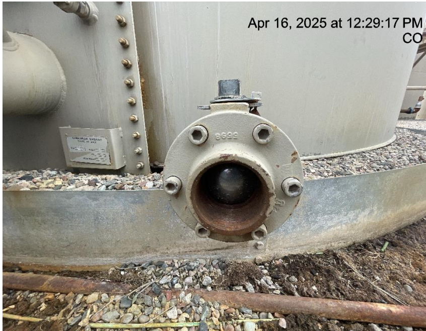
Photo # 1799 Open ended load line
