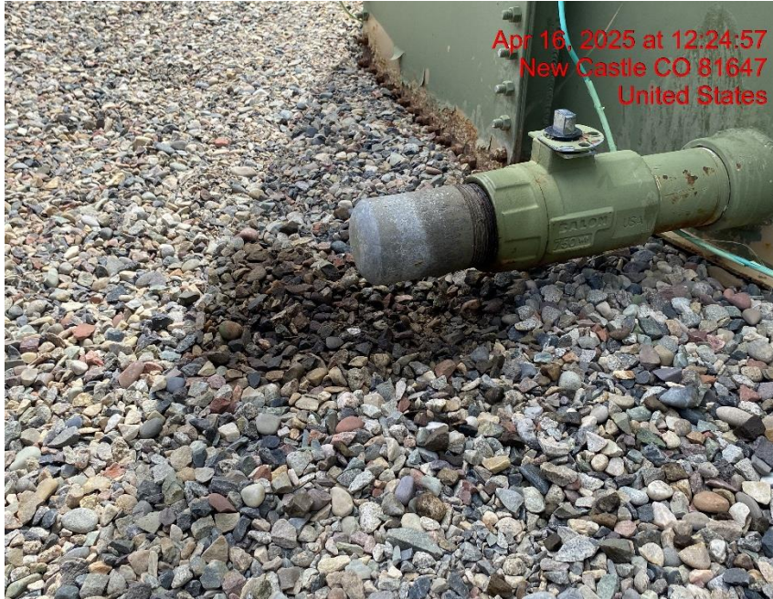
Staining in Tank Containment – Photo #08197
