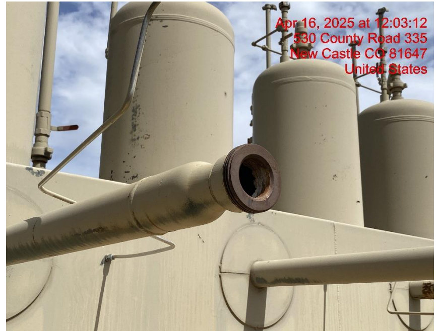
Wildlife Entry Hazard on Out-of-Service Separator – Photo #08159
