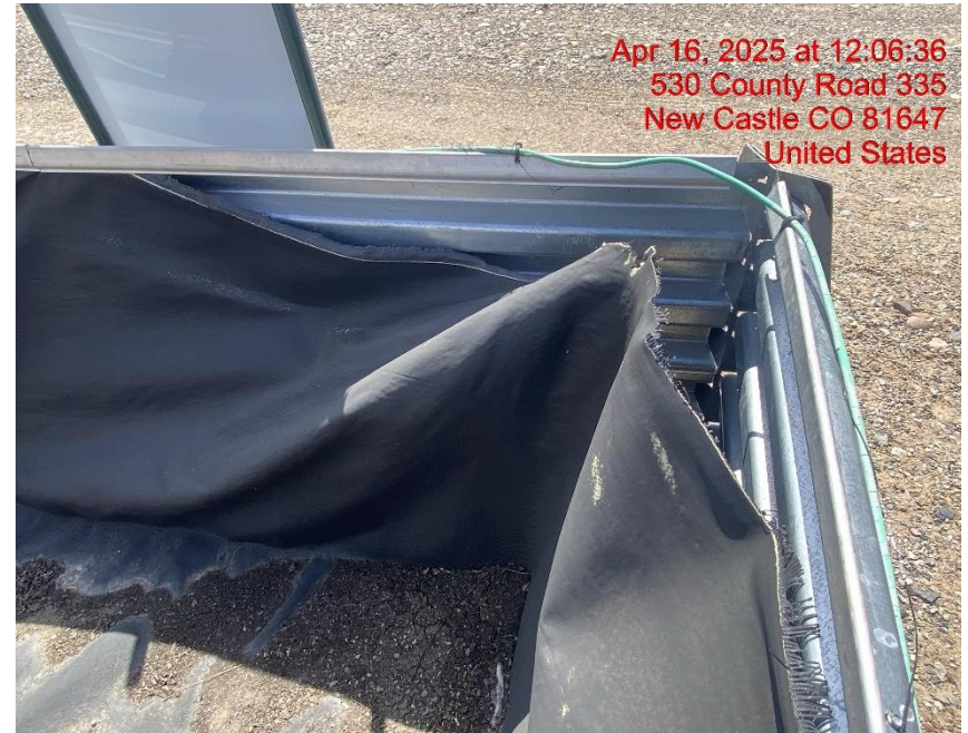
Damaged Berm Liner – Photo #08168
