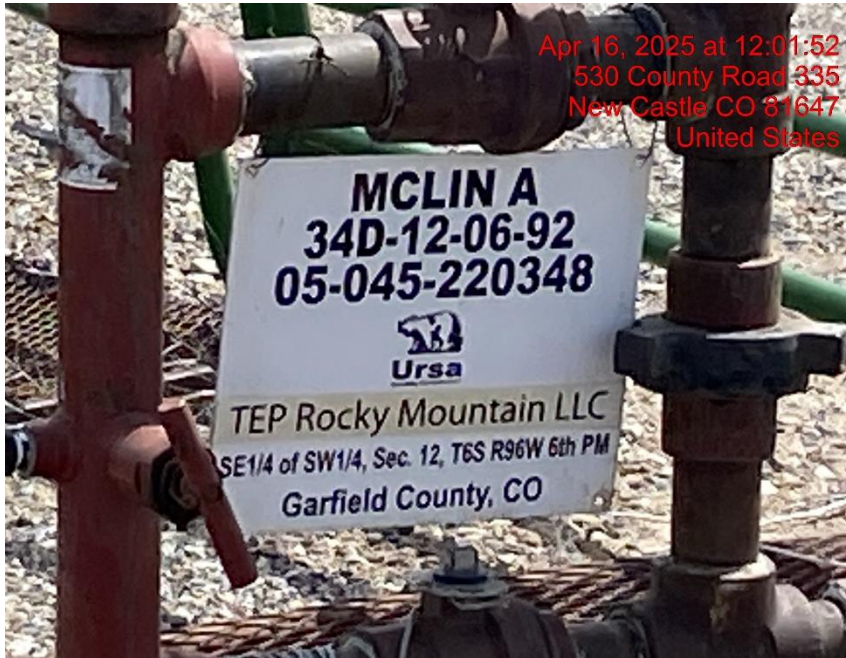
Inaccurate API Number on Wellhead Sign – Photo #08156
