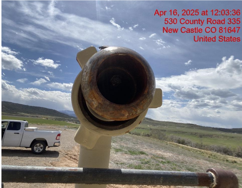
Wildlife Entry Hazard on Out-of-Service Separator – Photo #08160
