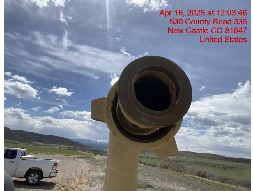
Wildlife Entry Hazard on Out-of-Service Separator – Photo #08161
