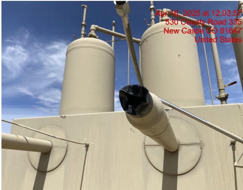
Wildlife Entry Hazard on Out-of-Service Separator – Photo #08162
