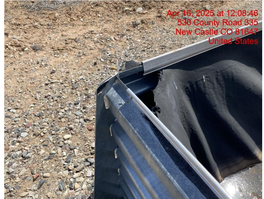
Damaged Berm Liner – Photo #08175
