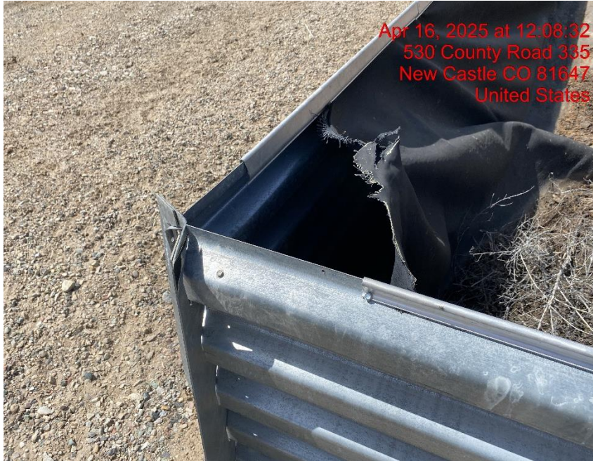
Damaged Berm Liner – Photo #08174
