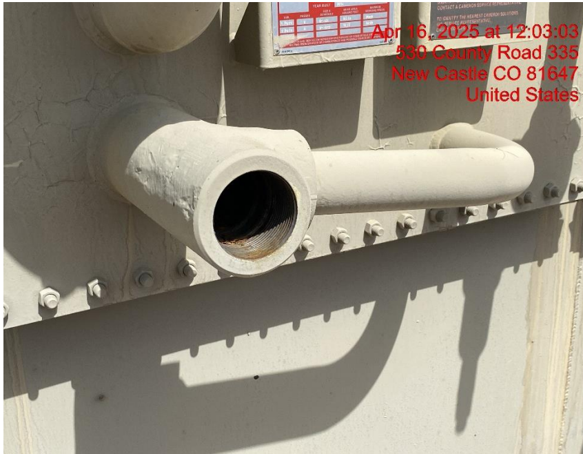
Wildlife Entry Hazard on Out-of-Service Separator – Photo #08158
