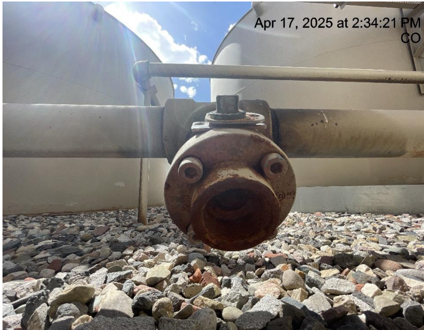
Photo # 2638 Open ended load line
