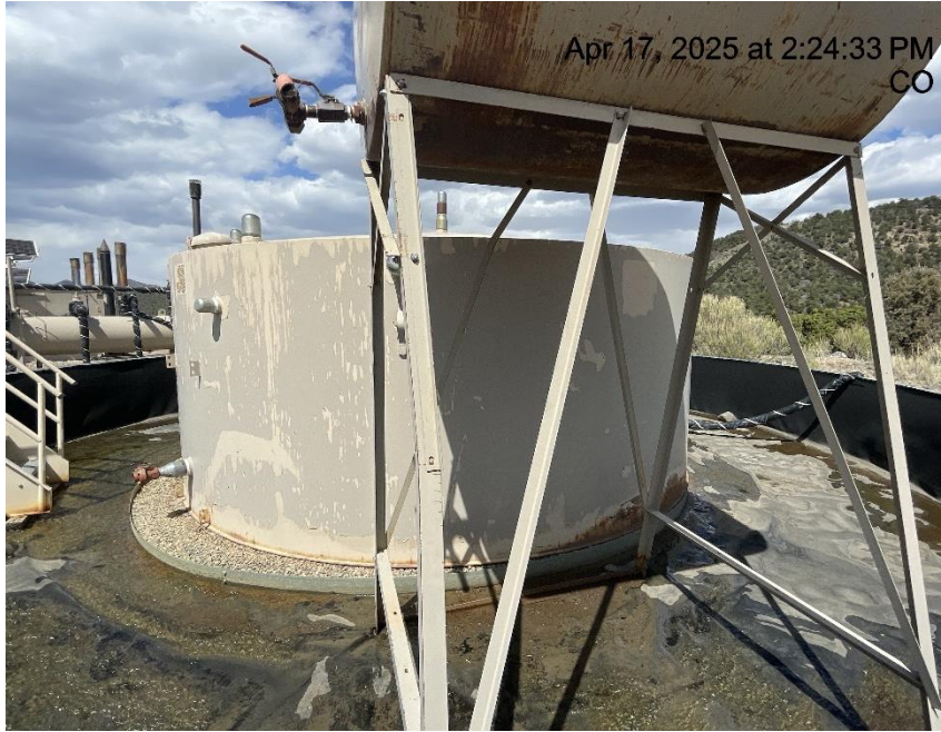
Photo # 2642 Arctictherm E-50 tank label lacks required information
