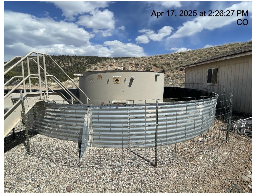
Photo # 2645 Labeling on methanol tank is weathered & some required information is illegible & additionally tank capacity is incorrect
