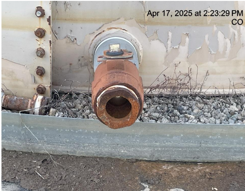
Photo # 2636 Open ended load line
