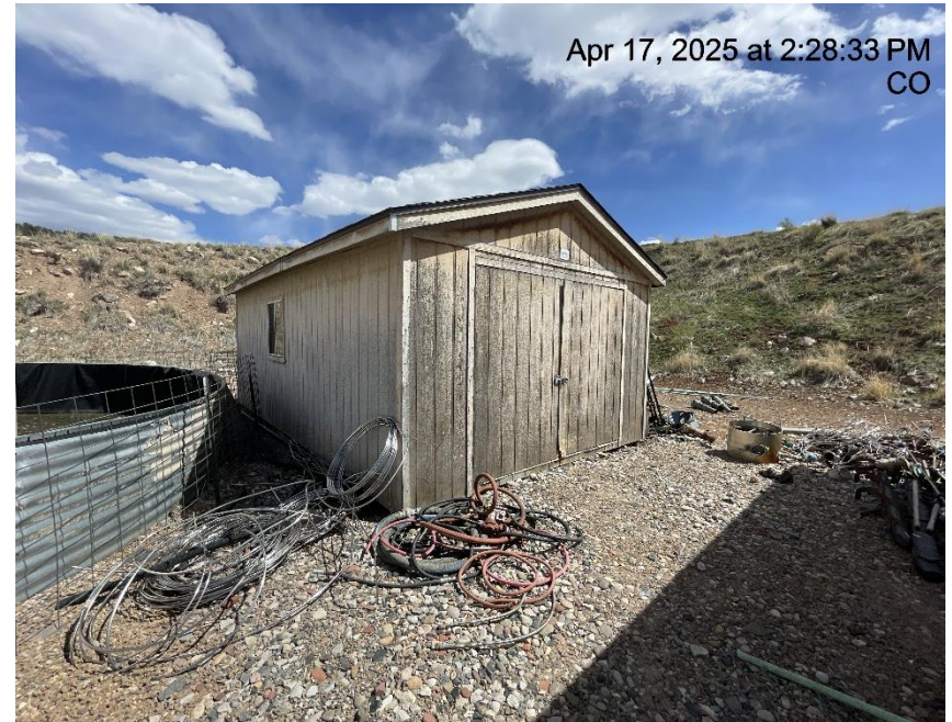
Photo # 2649 Shed on location/not in compliance with CECMC rules
