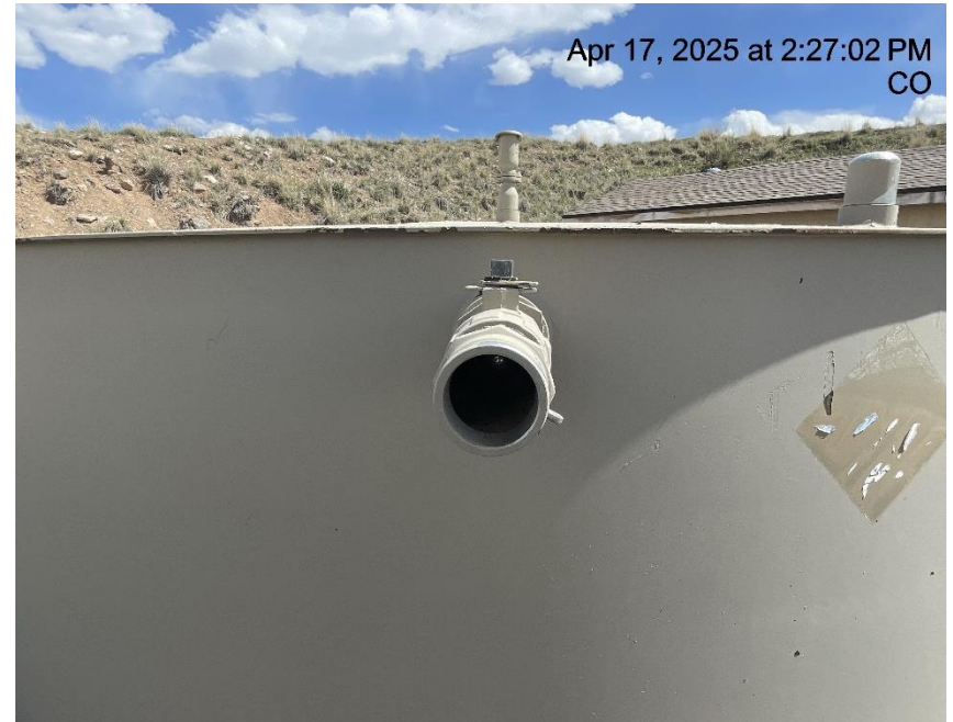
Photo # 2637 Open ended load line
