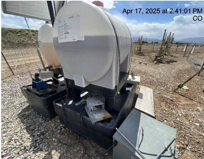
Photo # 2664 Unused chemical tank
