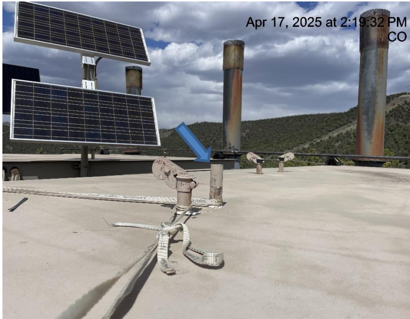
Photo # 2632 PRV vent line does not comply with CECMC pressure safety device rules
