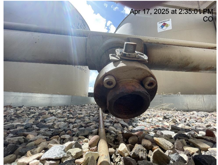
Photo # 2639 Open ended load line
