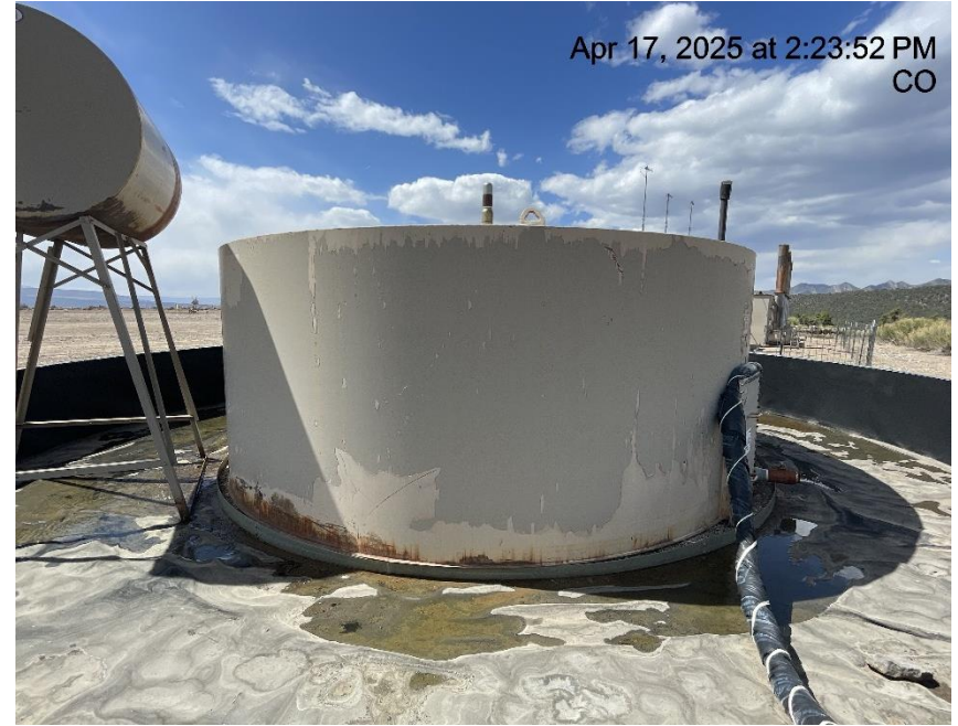
Photo # 2643 Arctictherm E-50 tank label lacks required information
