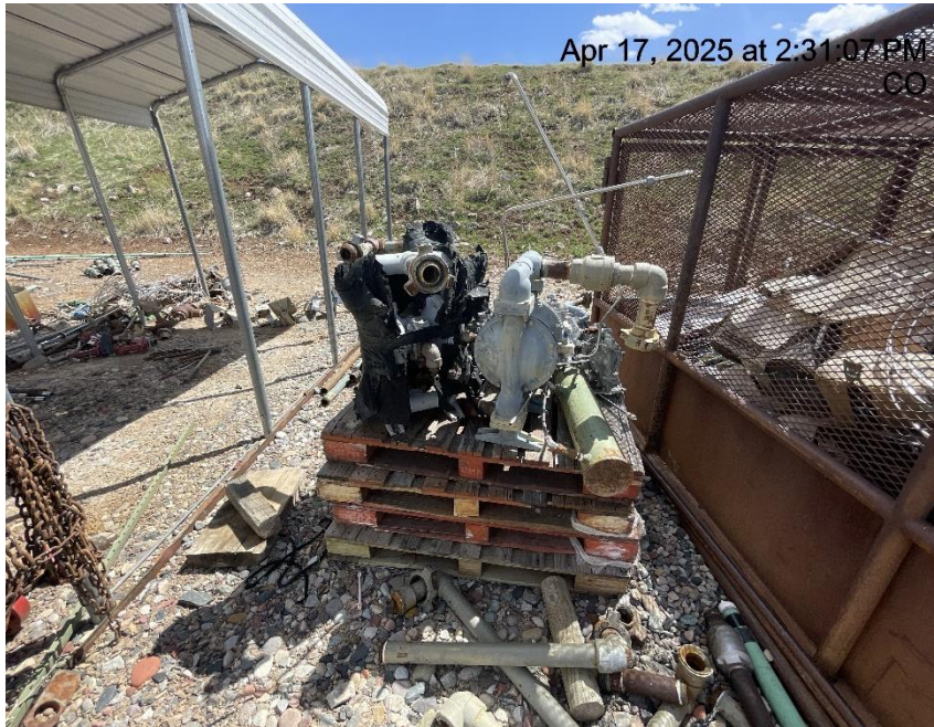
Photo # 2660 Unused pumps
