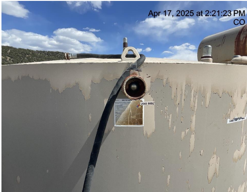
Photo # 2634 Open ended load line
