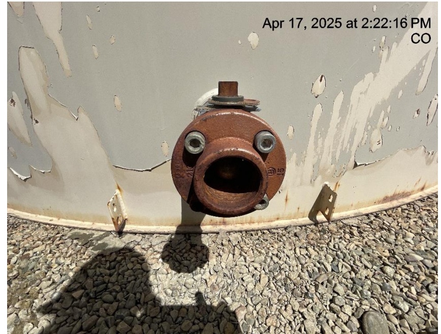
Photo # 2635 Open ended load line
