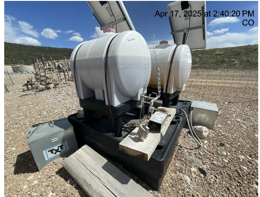
Photo # 2663 Unused chemical tank
