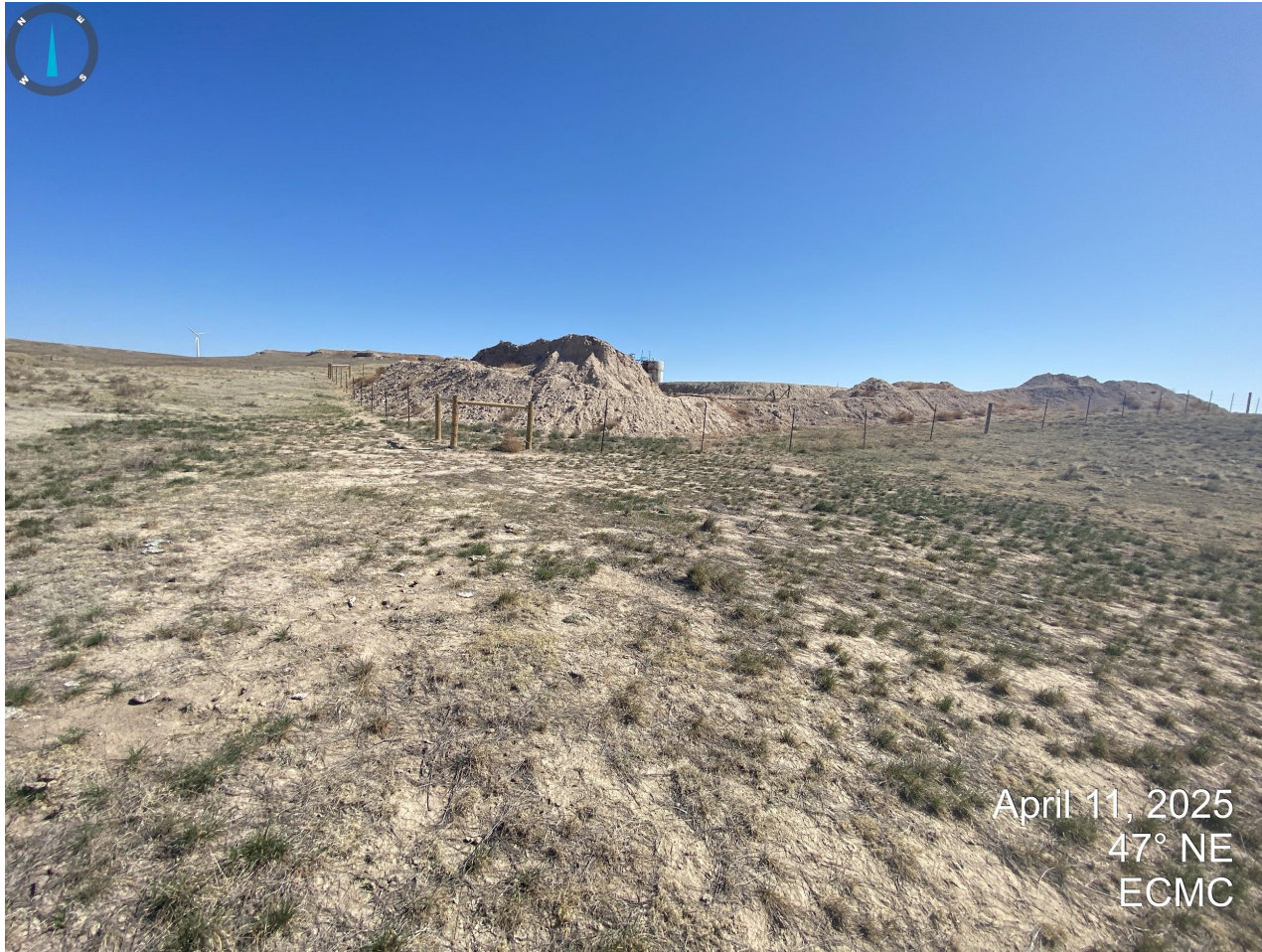
Photo 5. Sediment deposition resulting from unstabilized stockpiles, southwest corner of the pit.
