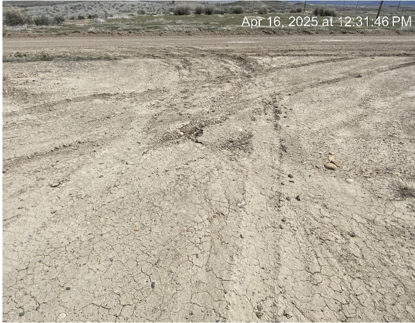
Entrance berm maintenance required
