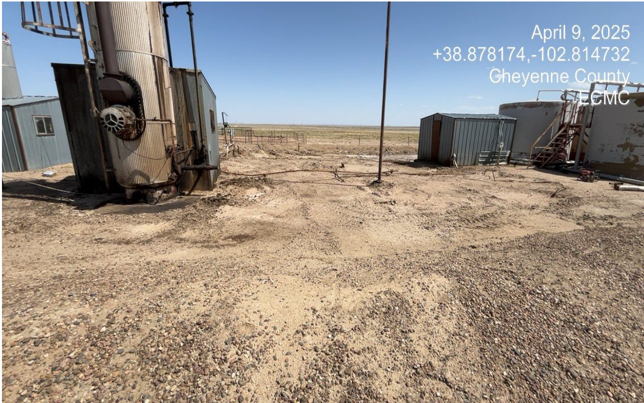
Photo 3. The previously observed that occurred near the heater treater. The surface and equipment was/is blackened from a hydrocarbon mist that occurred.
