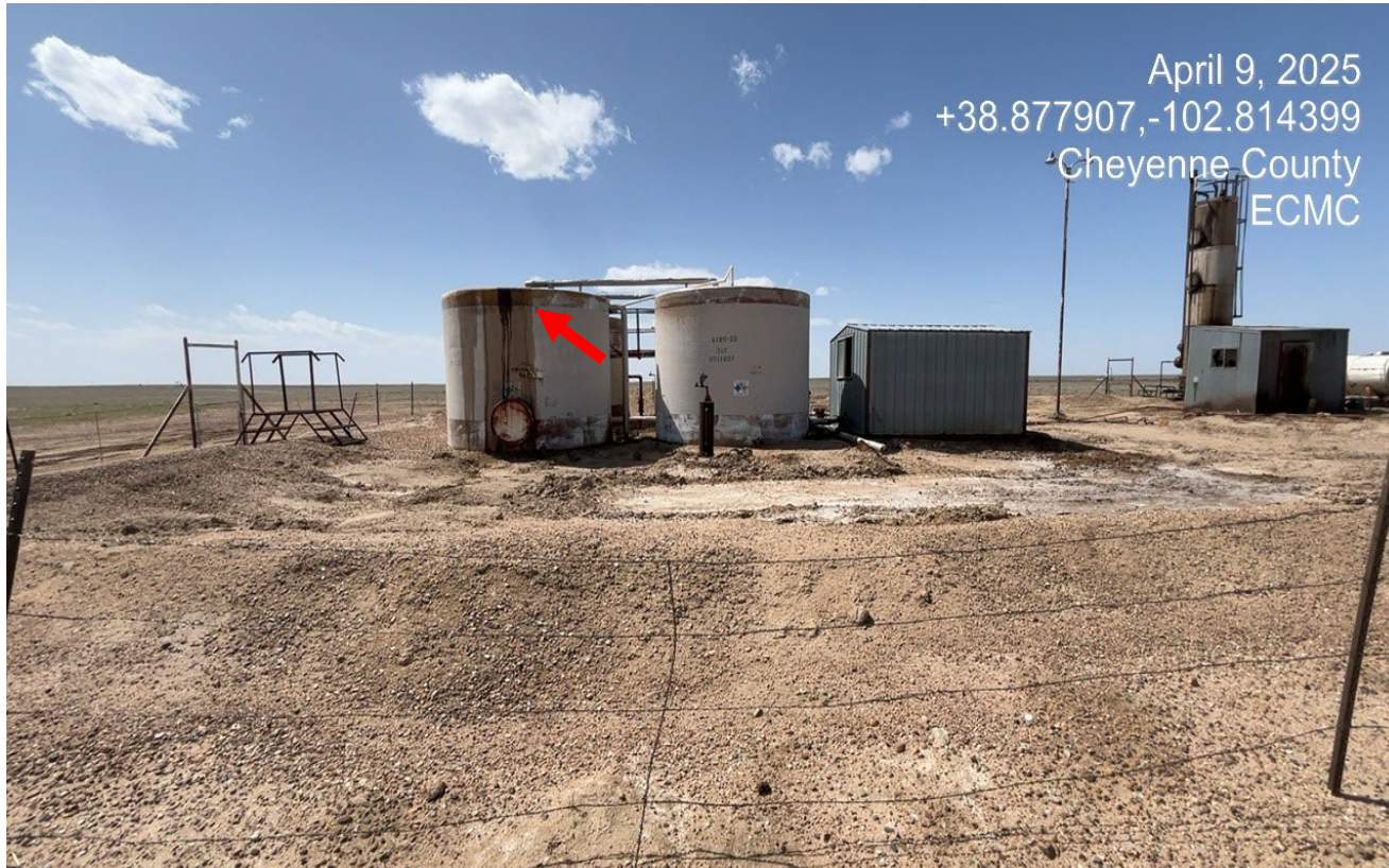
Photo 6. There are signs of a leak at the top of the fiberglass tank shown at red arrow.
