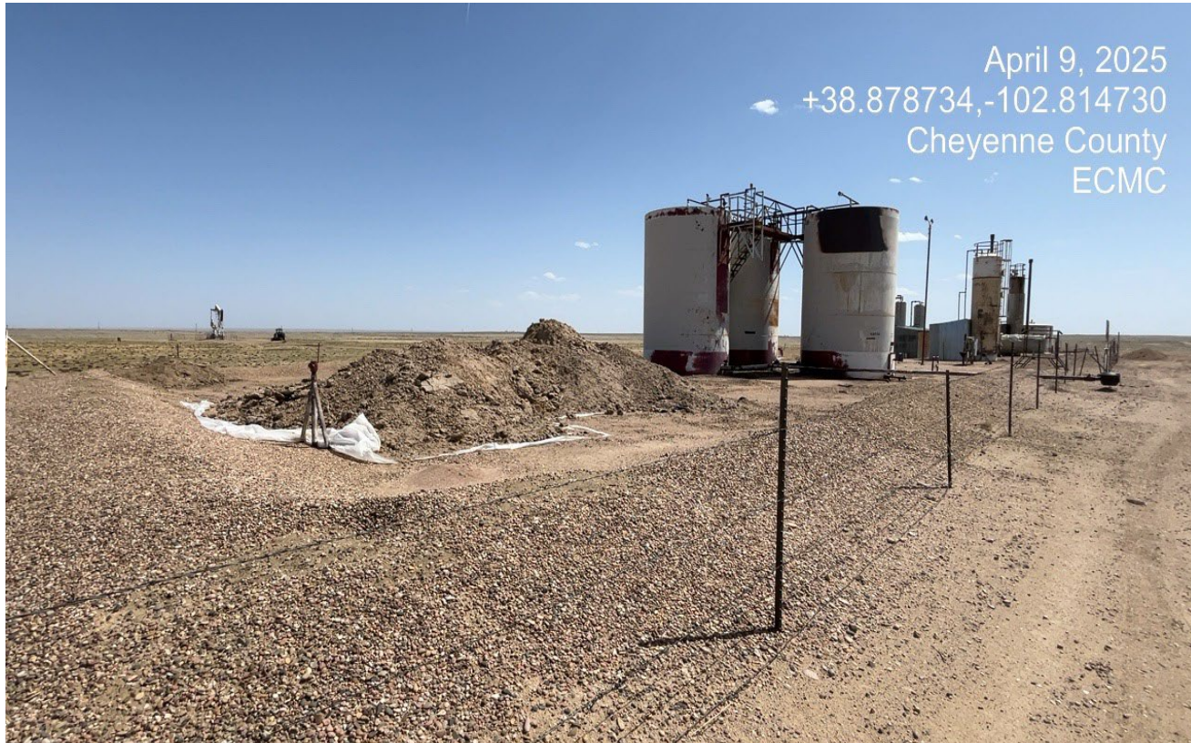
Photo 1. Facing southeast toward the tank battery. The E&P waste from the previously observed spill has been placed on a plastic liner at the north side of the tank battery.
