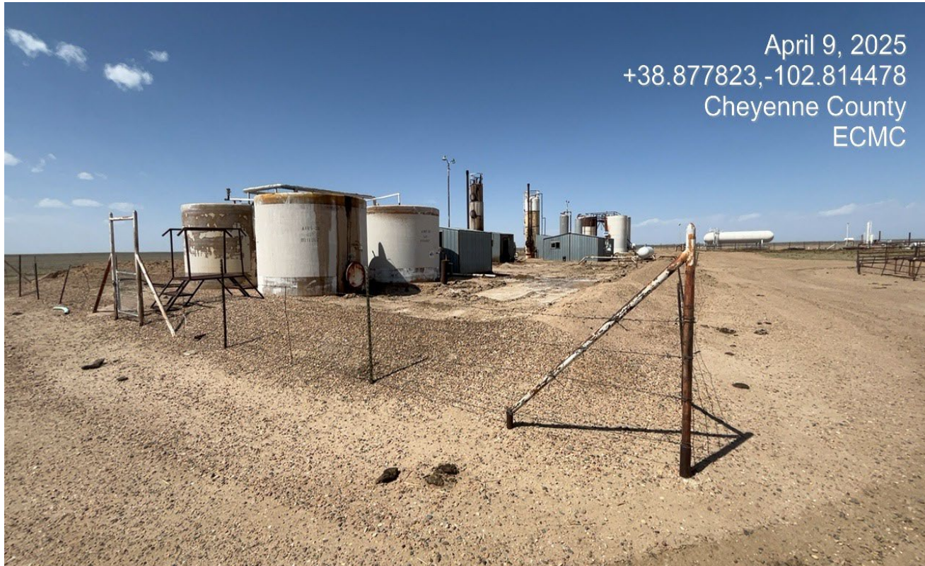
Photo 4. Southeast corner of the location facing northwest toward the tank battery facility. The previous spill had overtopped this corner with visible impacts shown in the previous inspection photos on 1/28/25.
