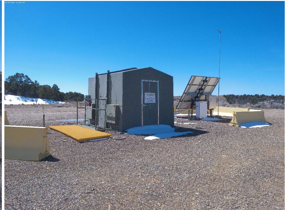
Injection Wellhead housing
